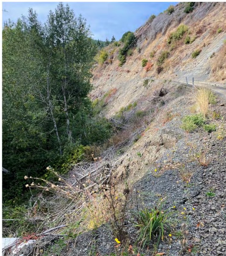
Figure 3. Example of a road segment with perched fill that presents a significant hazard to a fish-bearing stream.
