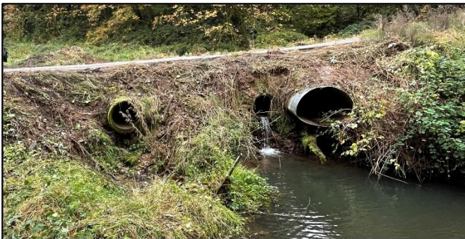
Before: Perched culvert restricting fish passage
