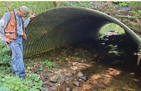
Culvert replacements like this one on Warner Creek (Astoria District) improve aquatic organism passage and restore habitat connectivity.
