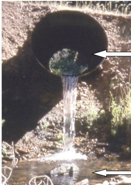
A. Perched culvert , as evident by the water drop.
