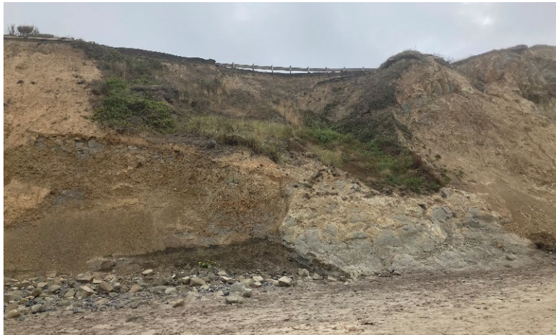
Figure 1. Exposed Guardrail Beach View
