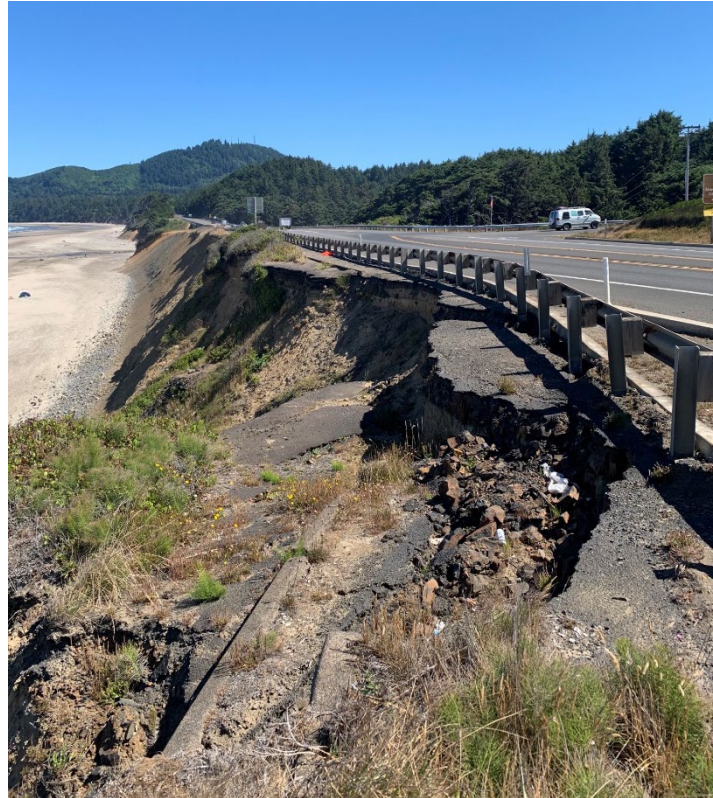
Figure 2. Highway Deterioration Street View
