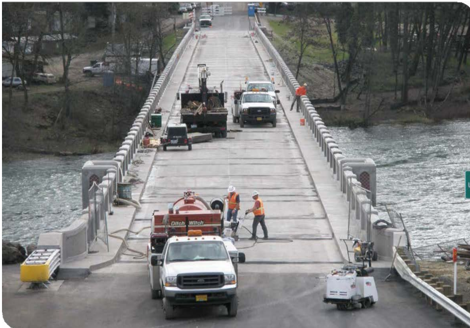
Winchester Bridge over the North Umpqua River (Roseburg, OR) – bridge rail and widening work (2008).
