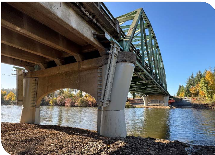
Coast Fork Willamette River Bridge - The truss span has been secured from falling off its supports.
