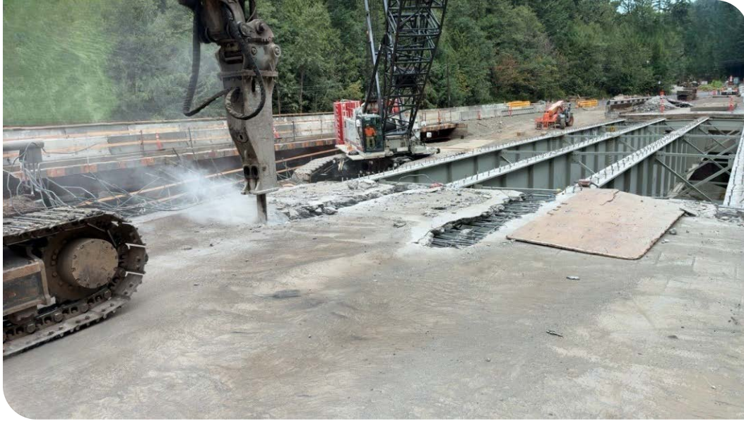
Salt Creek Bridge Replacement - Demolition of the existing bridge clears the way for building the new bridge.
