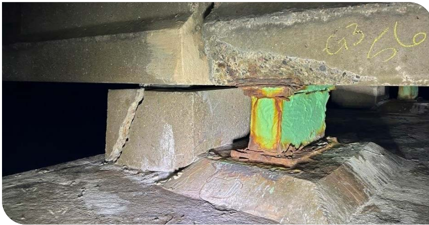
The photo left shows a corroded steel bearing and a cracked concrete support.
