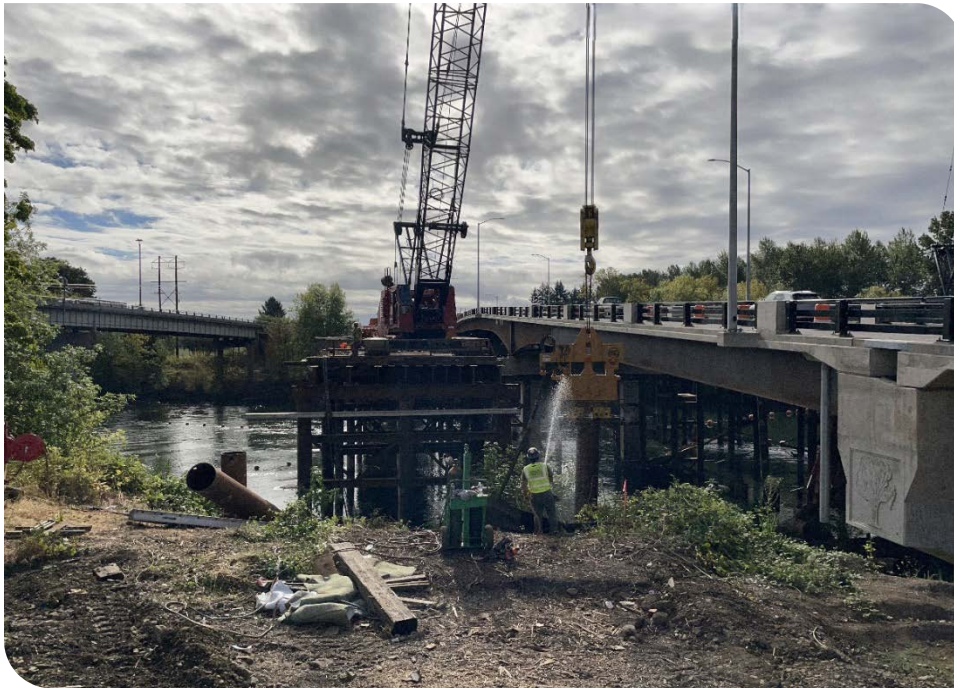
Van Buren Bridge – Traffic using the new bridge while work continues to remove the temporary structures.
