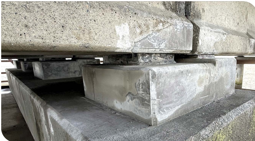
The photo left is an example of a completed repair on one of four cracked concrete supports on the Astoria-Megler Bridge
