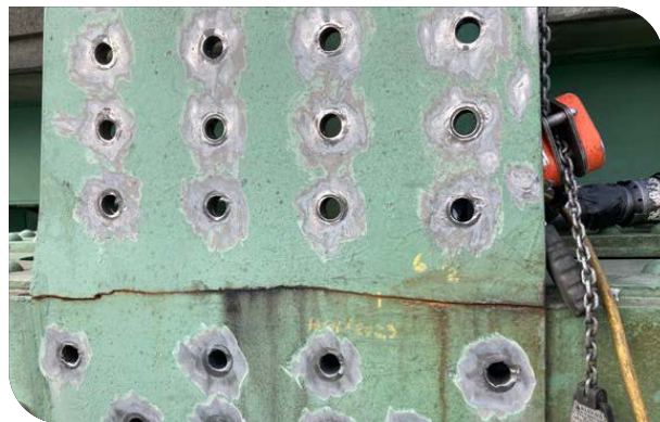
Steel Fatigue Crack
