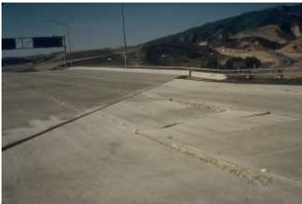
Case 3 (Photo courtesy of Caltrans)
