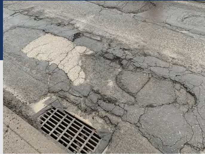
Road failing over existing storm sewer
