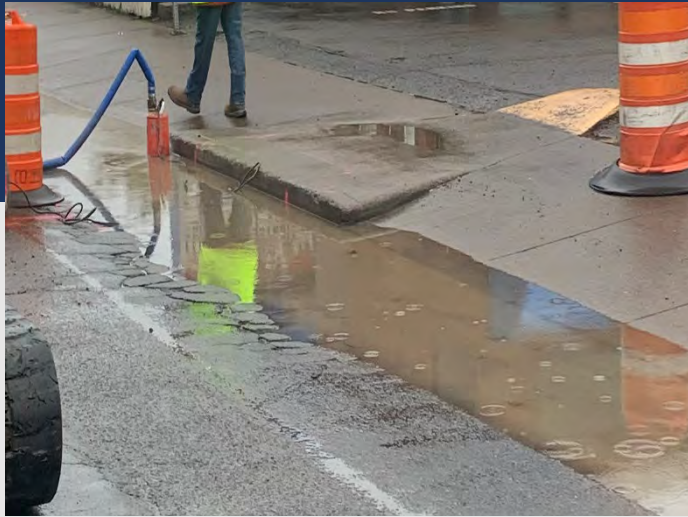
Water ponding along mainline
