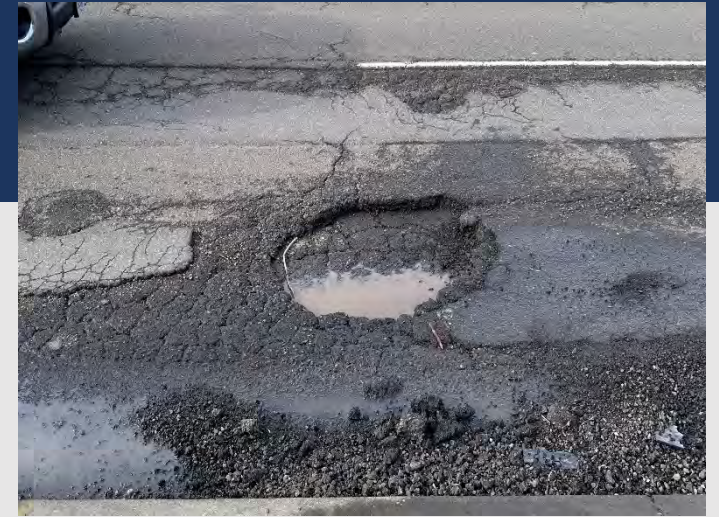
Deep potholes forming
