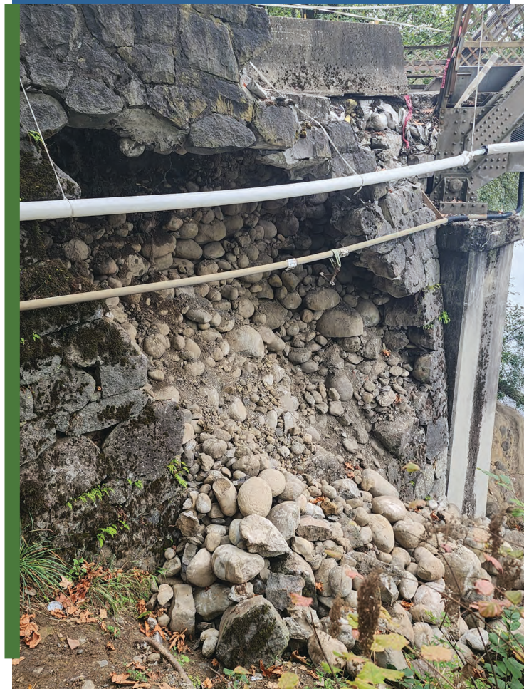
Photo showing retaining wall collapse prior to a recent 6-month emergency repair
