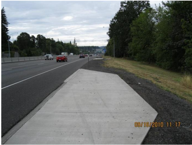
example of photo 8 facility access pad (concrete pad next to underground stormwater vault)
