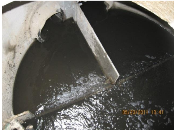
Example of photo 4A Flow splitter manhole (manhole located at the west corner of facility)
