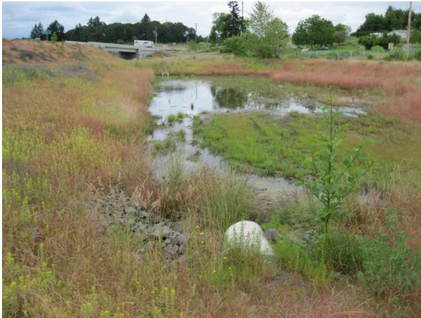
Example of photo 4 Facility inlet (inlet pipe located at bottom of photo)
