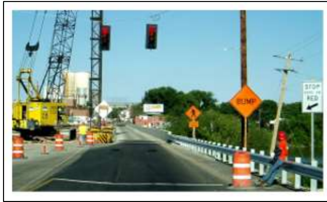
Figure 2-22: Temporary Traffic Signal (Span Wire)
