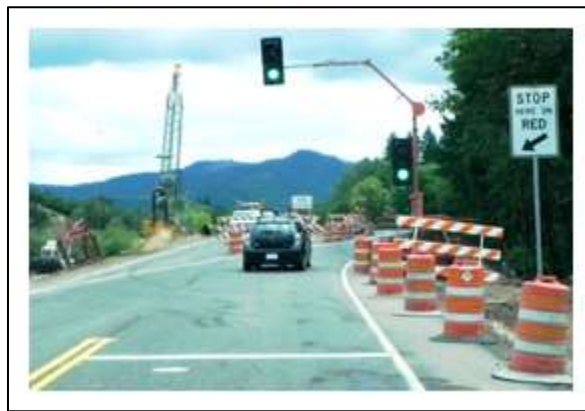
Figure 2-23: Portable Traffic Signal
