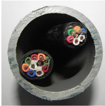
1 1/2" conduit w/control cables Does NOT exceed NEC max fill Exceeds ODOT max fill
