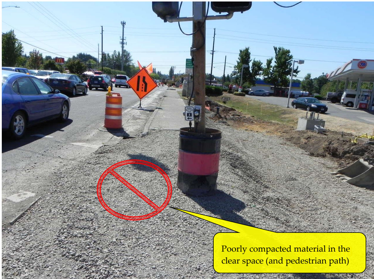
Figure 5-70 | Poorly Compacted Material Example
