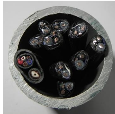
1 1/2" conduit w/9 loop feeder cables + 1 video cable Exceeds NEC max fill Exceeds ODOT max fill
