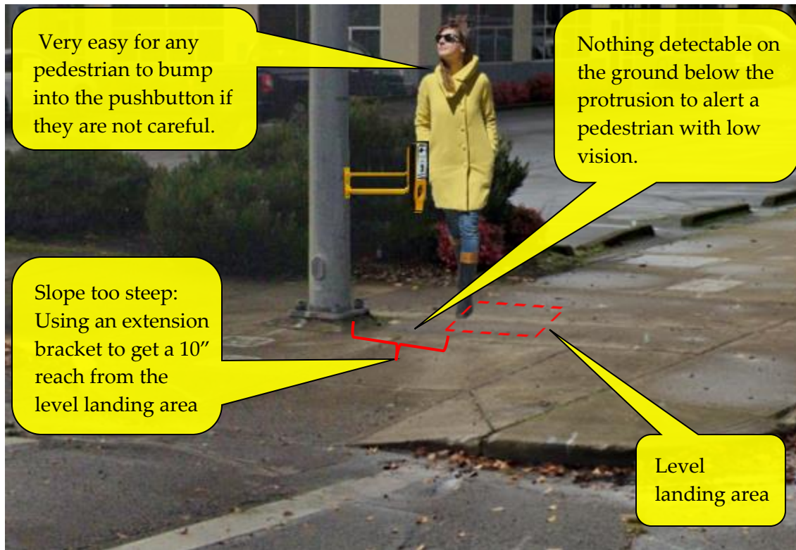
Figure 5-93 | Extension Bracket Mount Photoshop Example – Extending More Than 4 Inches into the Pedestrian Circulation Path
