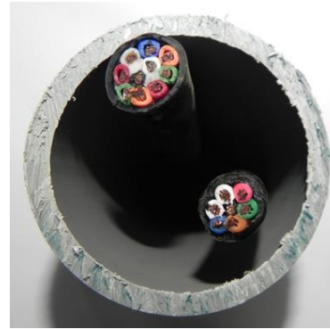
2" conduit w/control cables Does NOT exceed NEC max fill Does NOT exceed ODOT max fill
