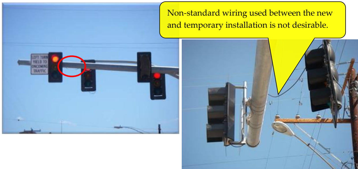
Figure 11-5 | Use of New Equipment for a Temporary Installation – This Practice Not Allowed
