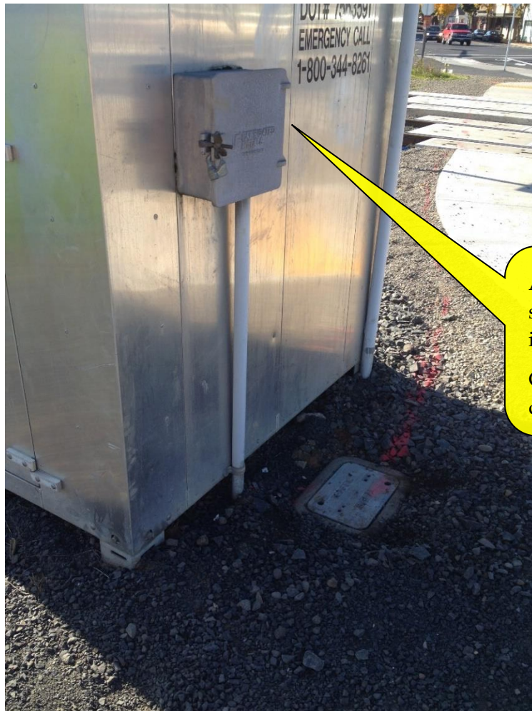
Figure 16-30 | Railroad Bungalow Access Box for Interconnect Conduit and Wiring
