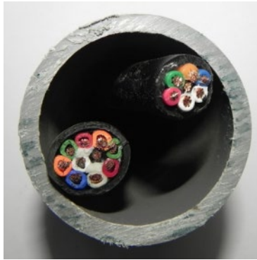
1 1/2" conduit w/control cables Does NOT exceed NEC max fill Exceeds ODOT max fill
