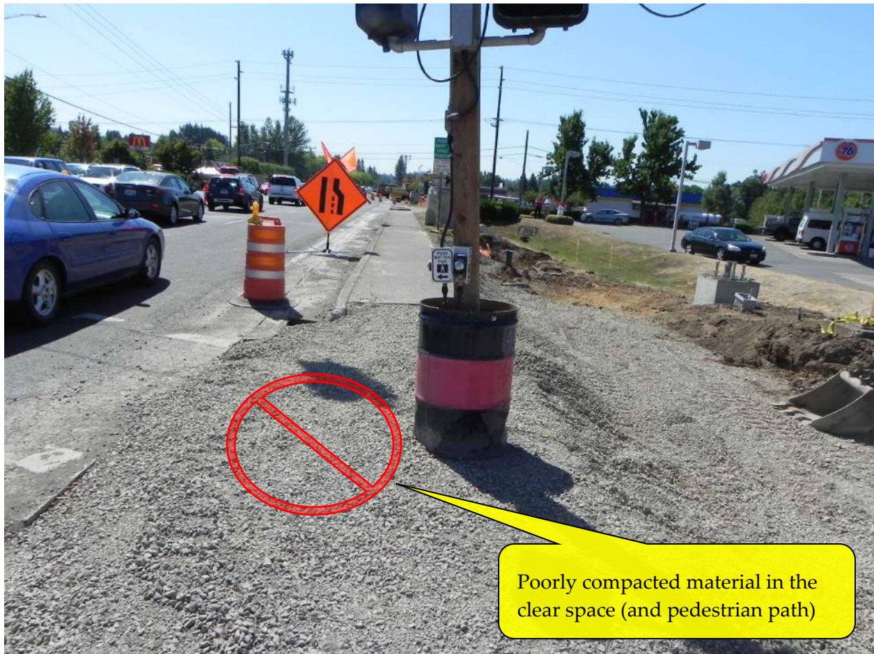
Figure 5-72 | Poorly Compacted Material Example
