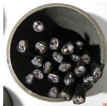
3" conduit w/22 loop feeder cables Does NOT exceed NEC max fill Does NOT exceed ODOT max fill
