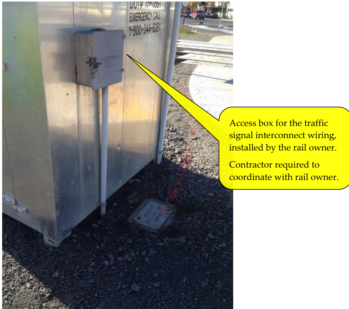
Figure 16-30 | Railroad Bungalow Access Box for Interconnect Conduit and Wiring
