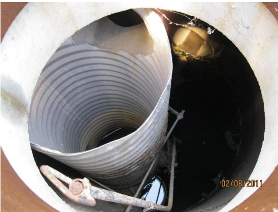
Example of photo 6A Flow control structure (flow control manhole located at east end of pond)
