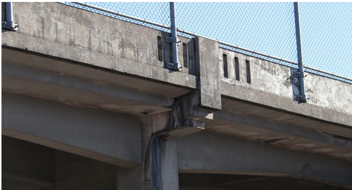
Photo 3: I-5 MP149.39 Equipment Overpass Bridge (Bridge #07643), showing “Three Bar” and protective screening detail, looking NE (taken 10/4/17 by Kenny Gunn)
