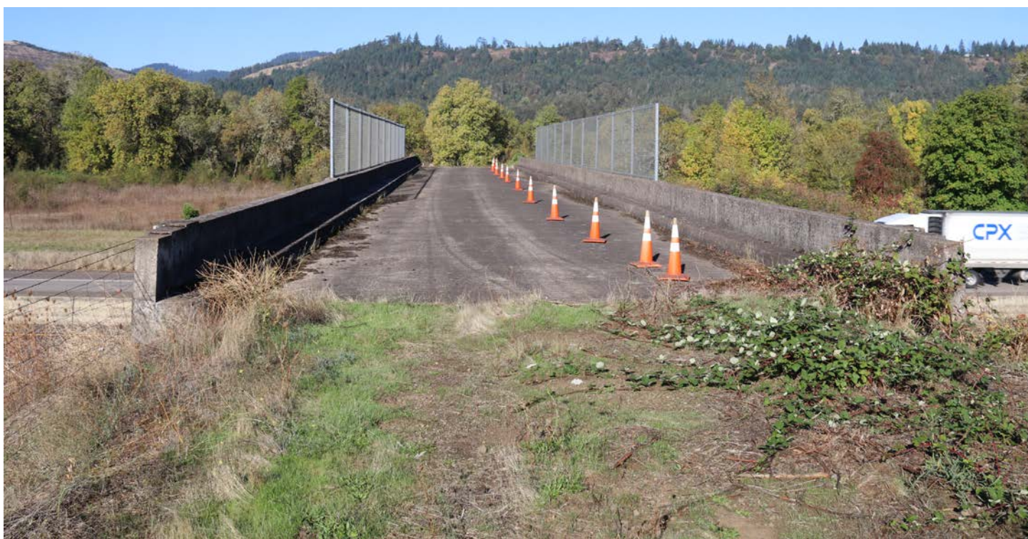
Photo 4: I-5 MP149.39 Equipment Overpass Bridge (Bridge #07643), looking West (taken 10/4/17 by Kenny Gunn)
