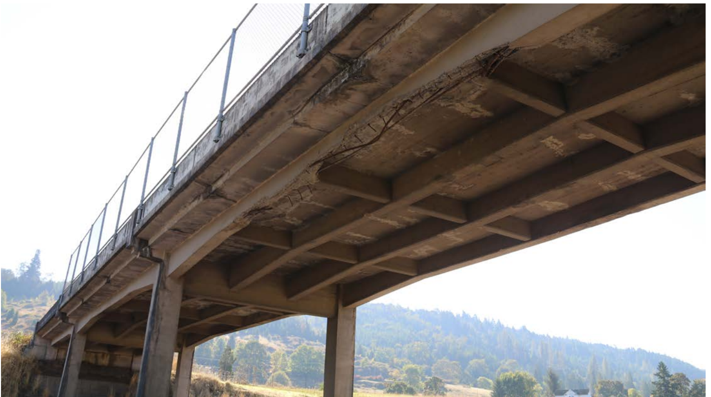
Photo 2: I-5 MP149.39 Equipment Overpass Bridge (Bridge #07643), showing underside of bridge and damage from large vehicles, looking SE (taken 10/4/17 by Kenny Gunn)
