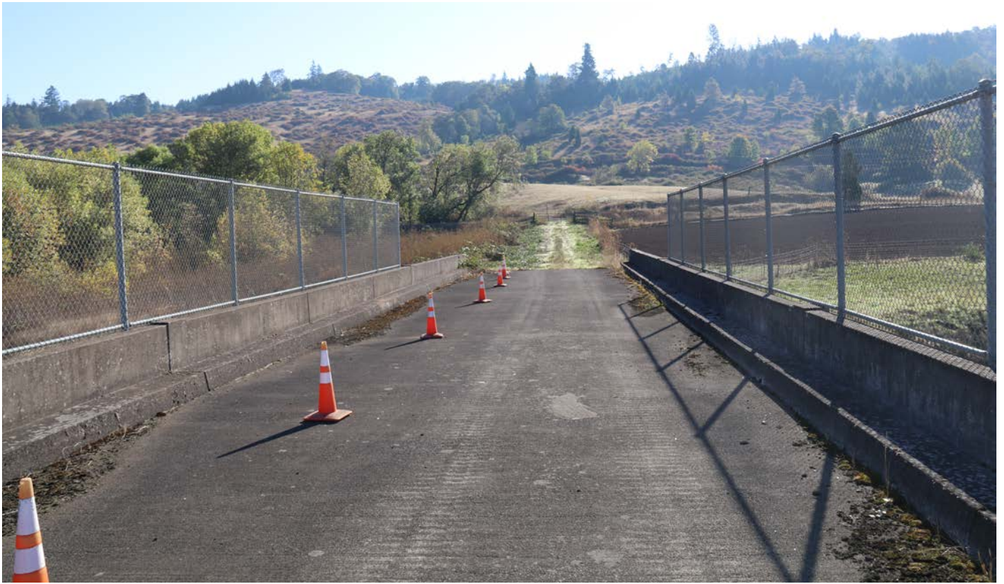
Photo 5: I-5 MP149.39 Equipment Overpass Bridge (Bridge #07643), looking East (taken 10/4/17 by Kenny Gunn)
