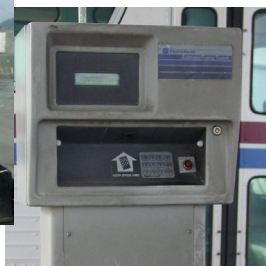
Fuel Tracking System
