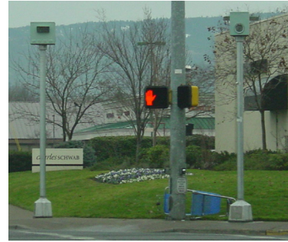
Photo Violation Detection at Biddle Road / McAndrews Road in Medford
