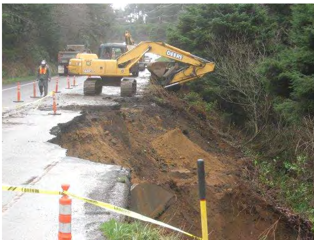
US101, January 19, 2012 slide – ODOT photo
