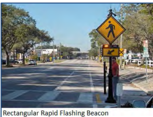
Rectangular Rapid Flashing Beacon
