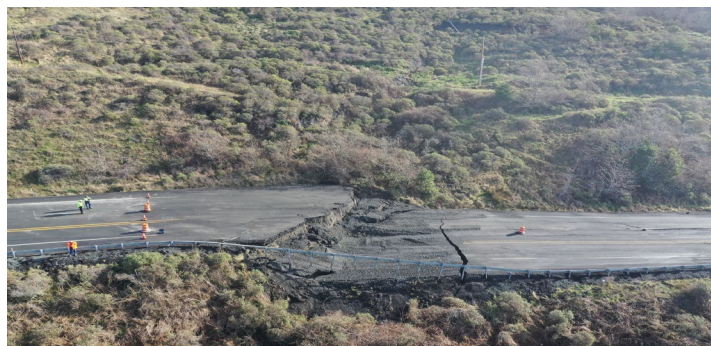
Figure 1: Arizona Inn landslide failure in Curry County closed Hwy 101 for nearly one week in January 2023 (ODOT, John Link)
