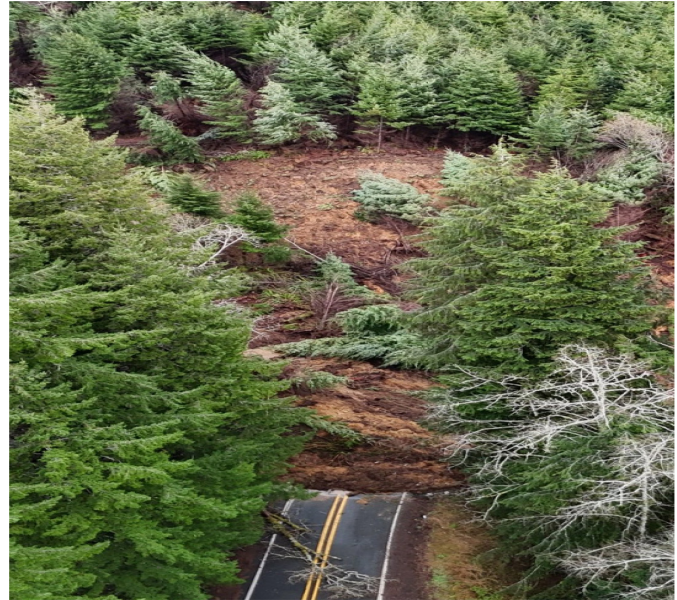
Figure 1: Recent Landslide closing Hwy229 (ODOT)
