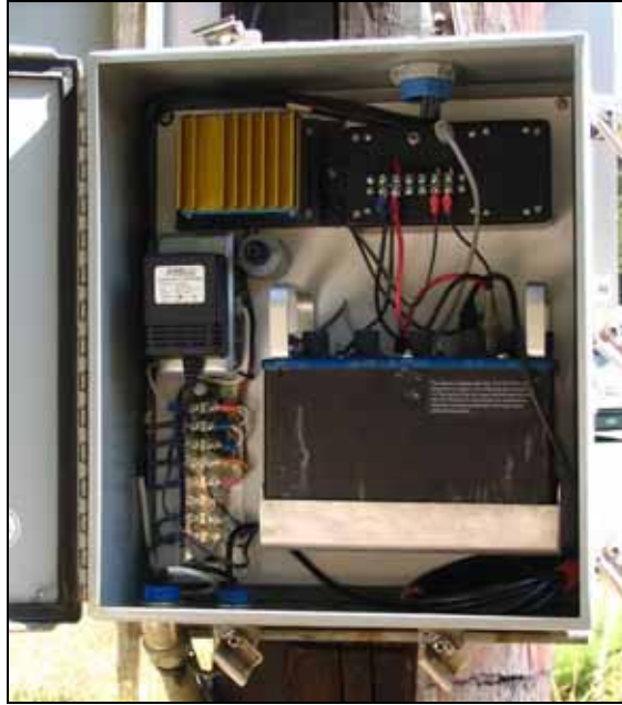
Figure 4.25: Cabinet with electronics for automated scanning for frequencies of radio collared elk and battery at one of the receiver stations in Sequim, Washington, USA (Photo: Marcel Huijser, WTI-MSU)
