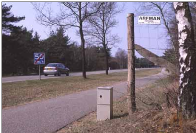
Figure 4.6: Cabinet with infrared sensor in 't Harde, The Netherlands (Photo: Marcel Huijser/WTI-MSU)
