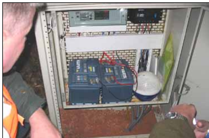
Figure 4.8: Control cabinet in 't Harde, The Netherlands (Photo: Marcel Huijser/WTI-MSU)
