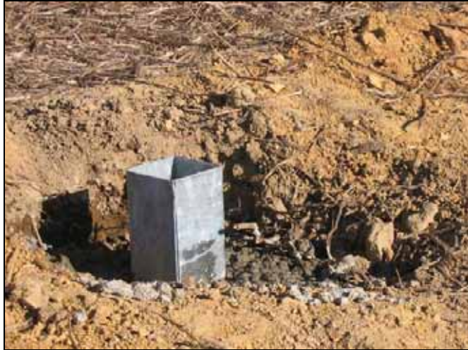
Figure 5.26: The wooden poles were fitted with a concrete foundation at the PA site (Photo: Marcel Huijser, WTI-MSU)
