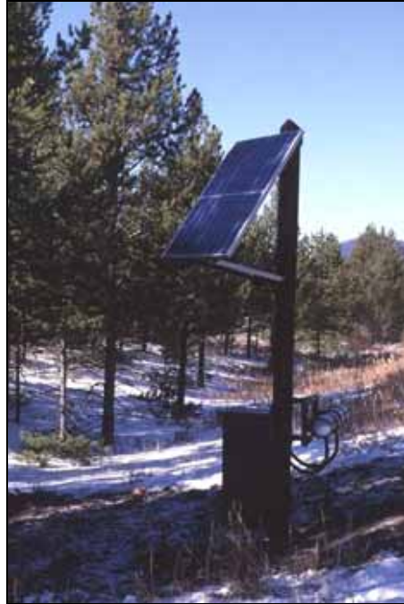
Figure 8.7: Care should be taken that solar panels are not placed in the shade of trees or other objects, including steep slopes. The angles of the sun should be calculated during winter, as daylight is scarce and the sun is low on the horizon. (Photo: Marcel Huijser, WTI-MSU)
