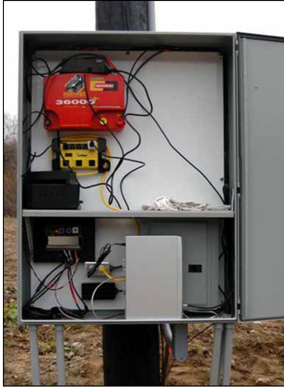
Figure 4.42: Control cabinet in Herbertville, Quebec, Canada. The upper section of the control cabinet contains the electronics for the electric fence; the lower section contains the electronics for the sensors and warning signals. (Photo: Ministère des Transports du Québec)
