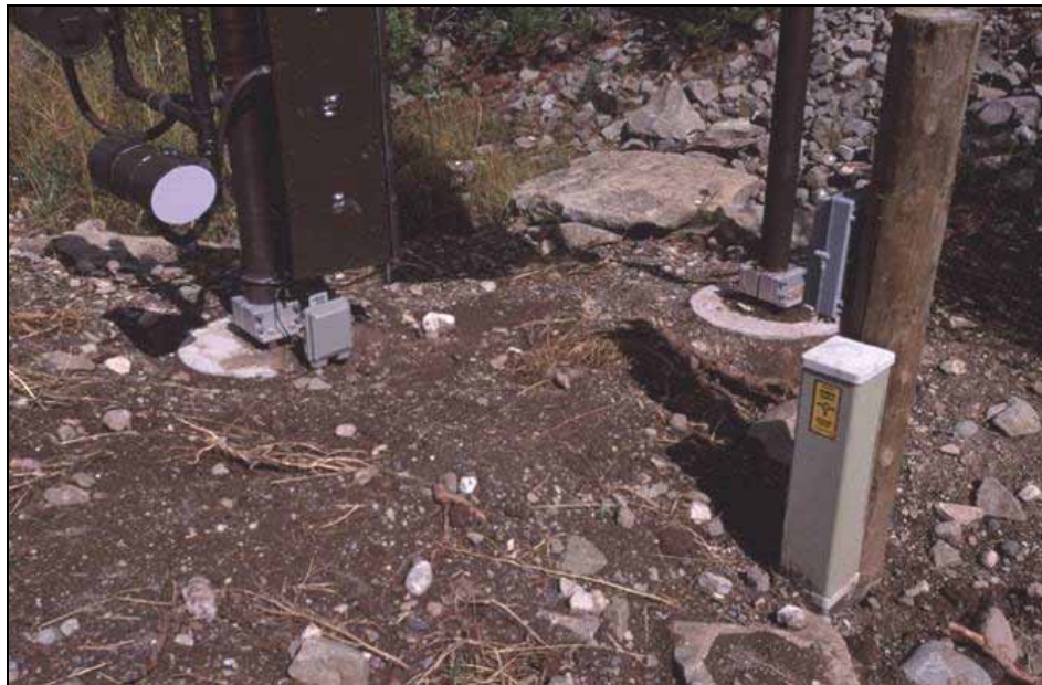
Figure 8.2: The problem with some of the concrete foundations was addressed by putting weed free soil around the posts while not blocking the drainage from the road. (Photo: Marcel Huijser, WTI-MSU)
