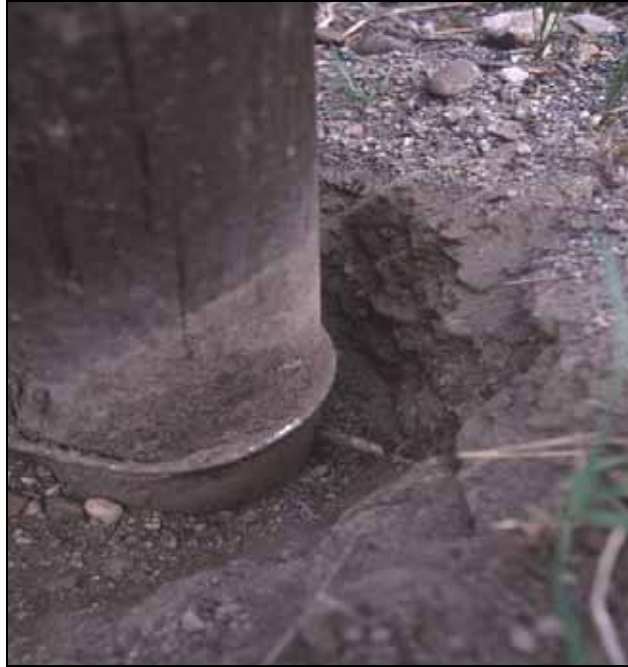
Figure 8.3: Some of the wooden poles were buried too deep. The stick indicates the upper of the three holes that serve as a break-away in case of a collision. All three holes should have been above the ground level. (Photo: Marcel Huijser, WTI-MSU)
