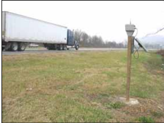
Figure 5.15: A station at the PA site. The sensors and battery are located inside the grey box on top of the pole. The solar panel is attached to the side of the pole. (Photo: Marcel Huijser, WTI-MSU)
