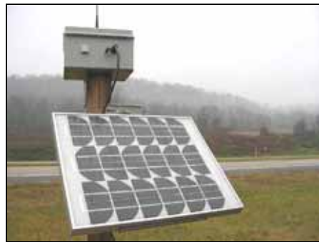
Figure 5.16: A closer view of the box with sensors, battery and the solar panel (Photo: Marcel Huijser, WTI-MSU)
