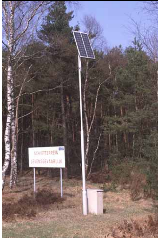
Figure 4.7: Solar panel and control cabinet in 't Harde, The Netherlands (Photo: Marcel Huijser/WTI-MSU)
