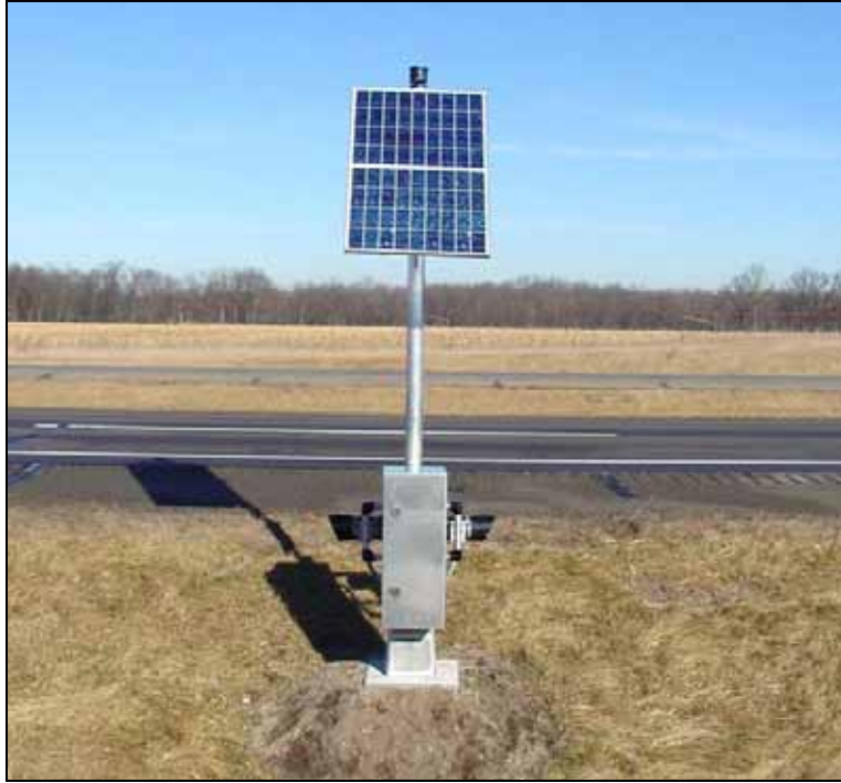
Figure 4.32: Pole with sensor tubes, cabinet (with circuit boards and batteries) and solar panel on the Indiana Toll Road, Indiana, USA (Photo: Indiana Department of Transportation, Toll Road District)
