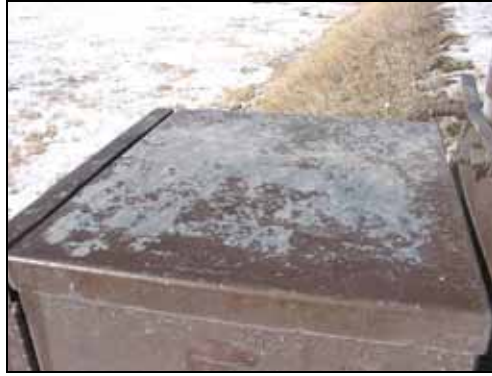
Figure 8.10: The elements can be hard on the equipment and the paint (Photo: Marcel Huijser, WTI-MSU)
