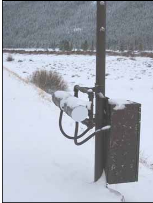
Figure 5.8: The sensors at one of the stations at the MT site. The cabinet contains a circuit board and batteries. (Photo: Marcel Huijser, WTI-MSU)
