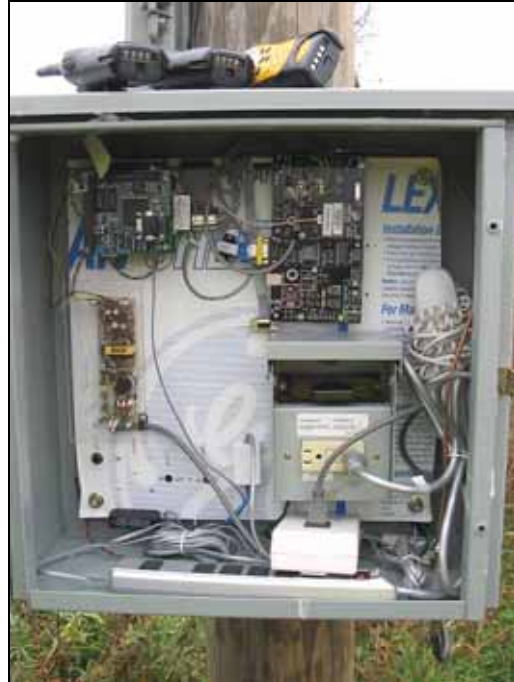
Figure 5.17: The control cabinet at the PA site (Photo: Marcel Huijser, WTI-MSU)
