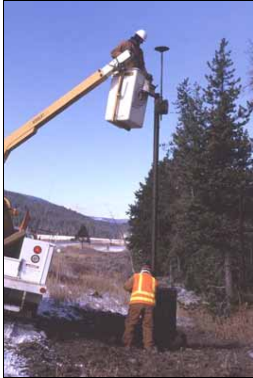
Figure 5.23: Installation of the antennas, beacons, signs and solar panels at the MT site required the use of a bucket truck (Photo: Marcel Huijser, WTI-MSU)
