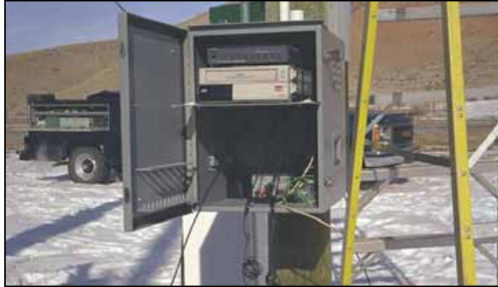
Figure 4.21: Video recorder system at Nugget Canyon, Wyoming, USA (Photo: Bill Gribble, WYDOT)
