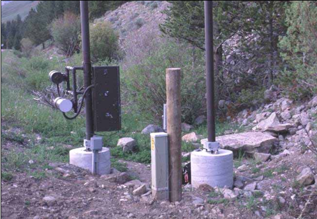
Figure 8.1: Some of the concrete foundations were in the clear zone and too high above the ground. This is the master station. The wooden post on the foreground is for the link to the land-based phone line. (Photo: Marcel Huijser, WTI-MSU)
