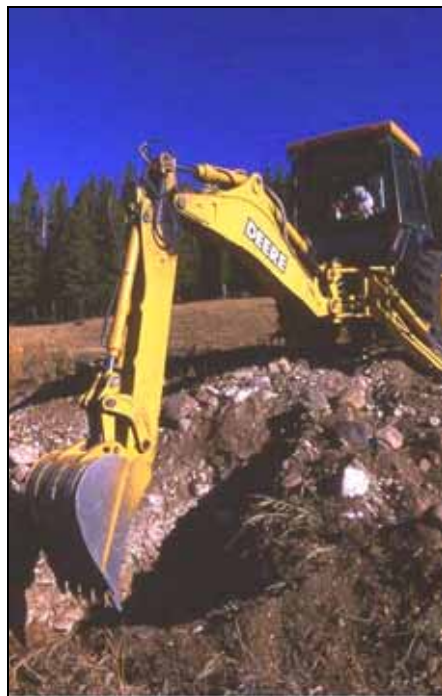
Figure 5.22: Eagle Rock Timber installed the poles and foundations at the MT site (Photo: Marcel Huijser, WTI-MSU)
