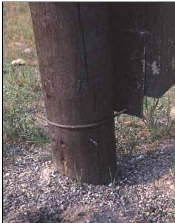
Figure 8.4: The problem with some of the break-away constructions for the wooden poles was addressed by drilling new holes at the appropriate height above the ground level. (Photo: Marcel Huijser, WTI-MSU)
