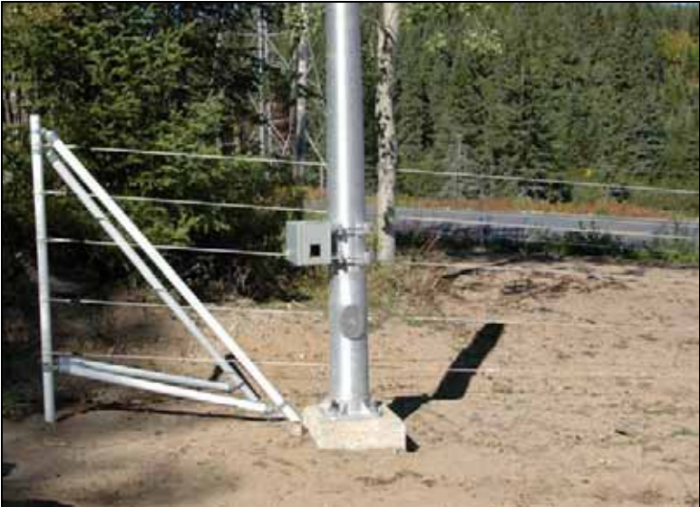
Figure 4.41: Sensor and electric fence in Herbertville, Quebec, Canada (Photo: Ministère des Transports du Québec)
