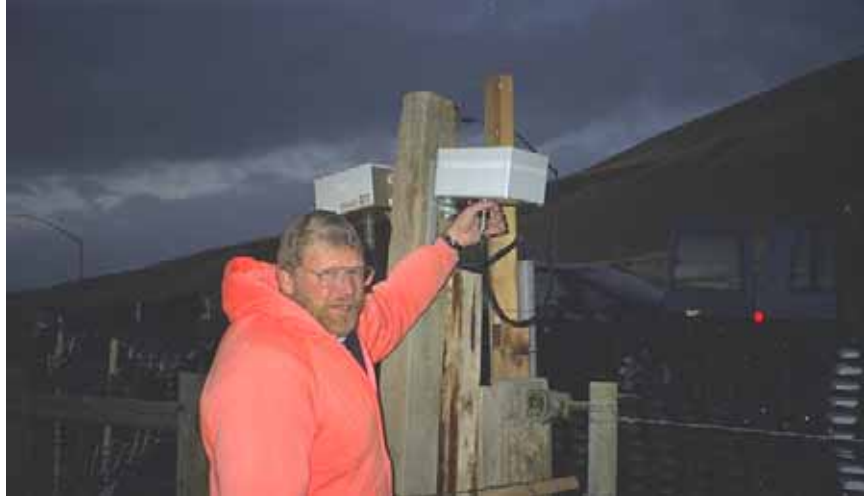
Figure 4.19: Microwave radar transmitters at Nugget Canyon, Wyoming, USA (Photo: Bill Moore, WYDOT)
