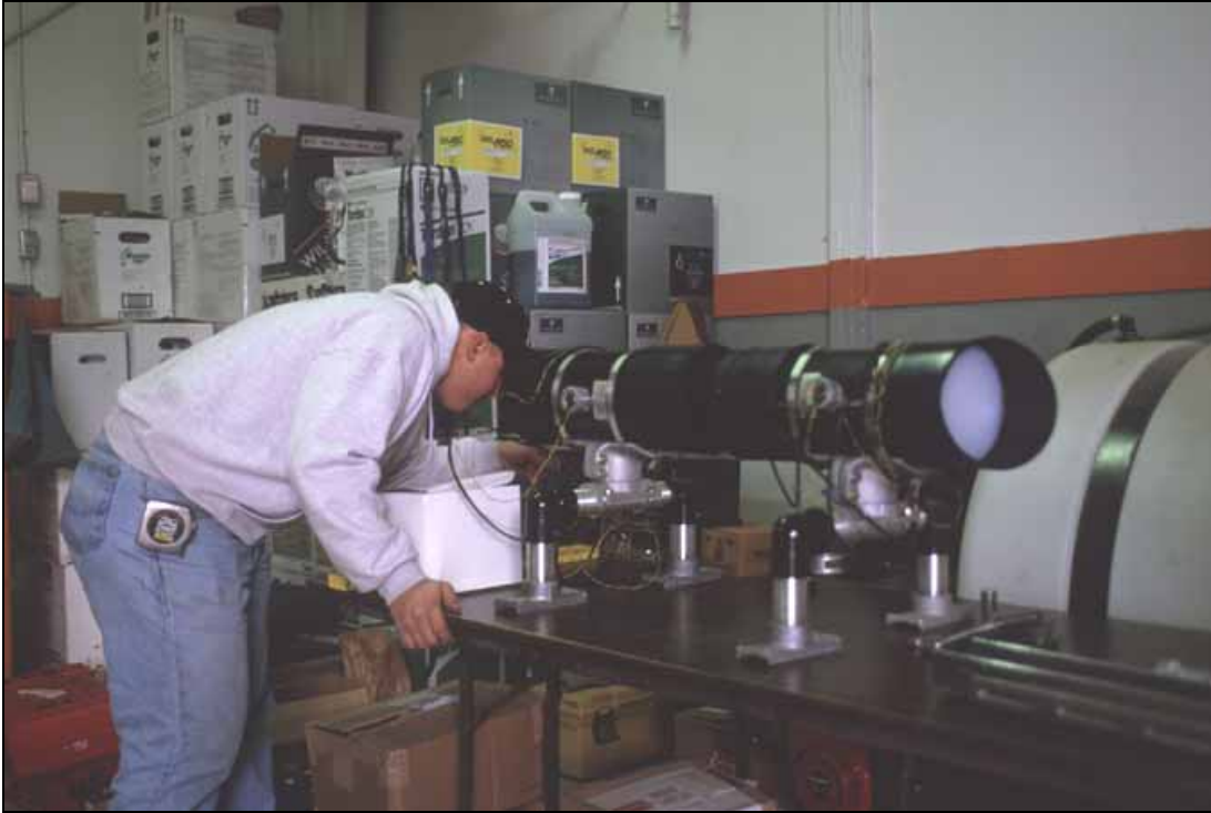
Figure 5.21: Michiana Contracting, Inc. assembled the animal detection system at the MDT maintenance yard in Bozeman, MT (Photo: Marcel Huijser, WTI-MSU)
