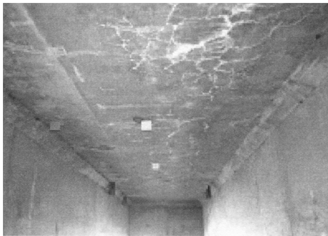
Figure 7.2: Typical cracking and damage visible on deck soffit
