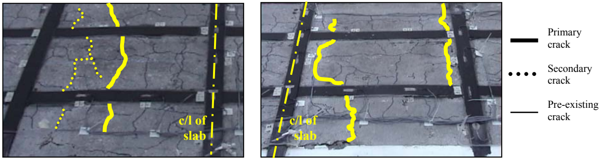
Figure 9.12: Crack pattern in Slab 3
