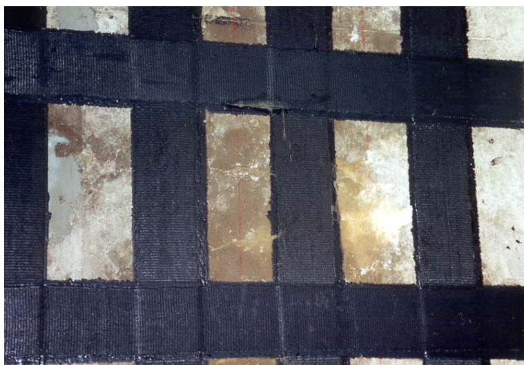
Figure 7.A5.9: Occurrence of damp patches on soffit
