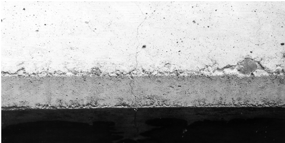
Figure 7.A5.5: Crack propagation through bottom face of girder
