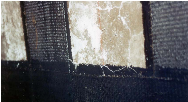
Figure 7.A5.3: Crack propagation in region between composite strips and through the primer
