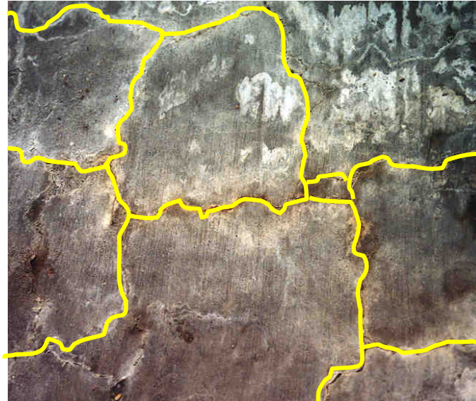
Figure 7.4: Crack pattern in soffit showing Stage 3 cracking
