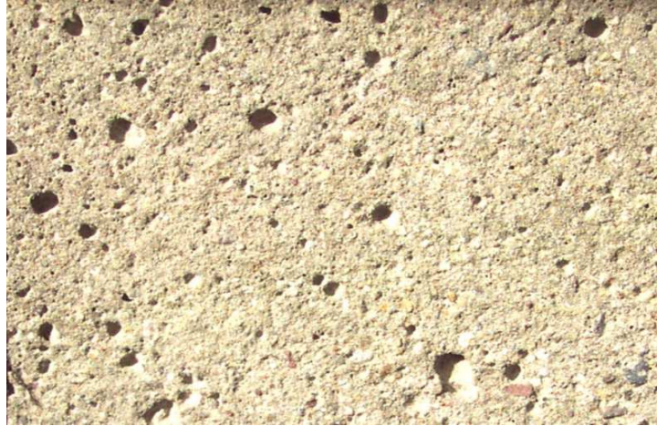
Figure 2.18: Concrete surface irregularities
