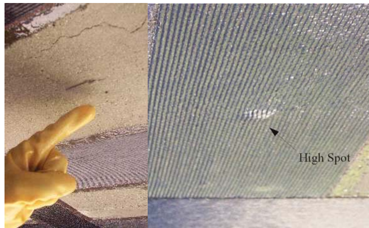
Figure 2.23: Air entrapment over high spots
