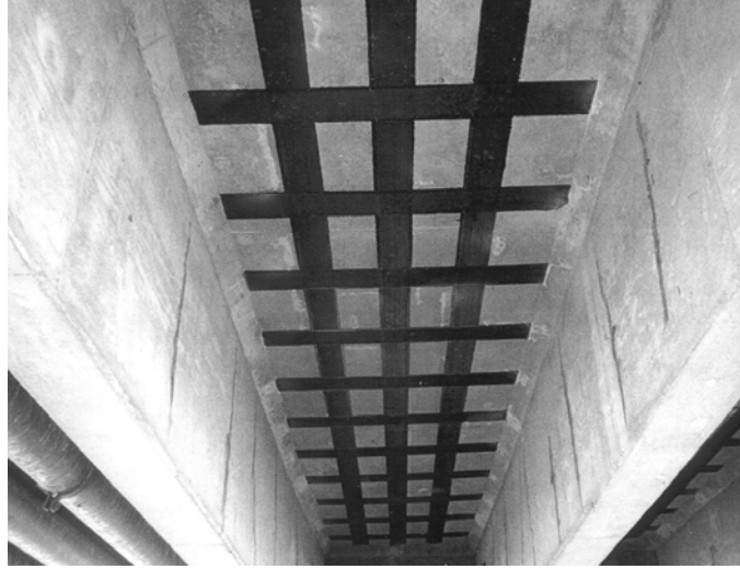
Figure 7.6: Example of strengthening through the use of field impregnated (wet layup) unidirectional fabric
