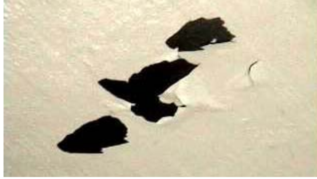
Figure 2.39: Damaged surface coating
