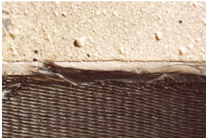
Figure 2.34: Pullout of loose fiber during infiltration
