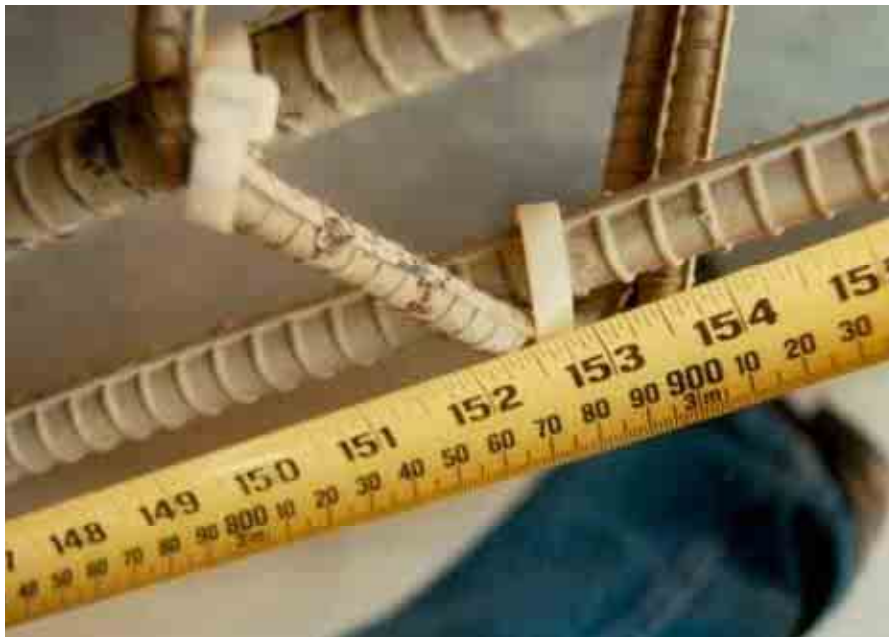
Figure 3.6: Corrosion Along a #3 Hoop
