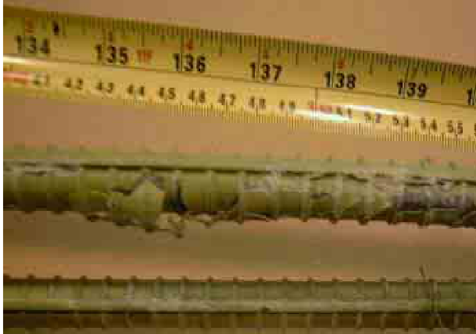
Figure 4.22: Disbondment of the Coating at the Tidal and Dry Zone Interface
