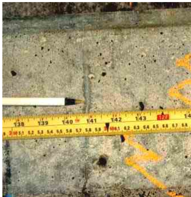
Figure 4.3: Transverse Cracking Propagated from the Reinforcing Hoop.
