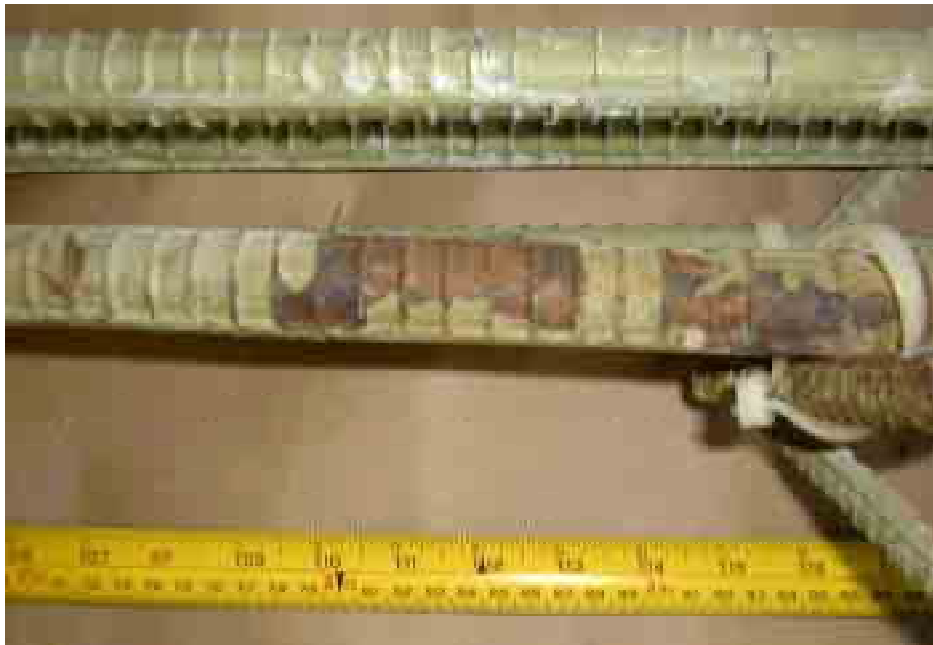
Figure 4.17: Corrosion Along Rebar #1 (2.8 to 2.95 m from bottom end of beam)
