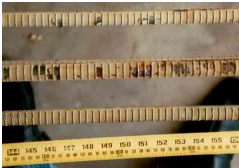
Figure 3.2: Corrosion Along the Longitudinal Bar
