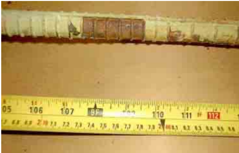
Figure 4.18: Corrosion Along Rebar #1 (2.75 m from bottom end of the beam)
