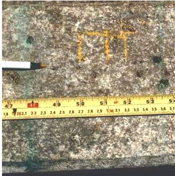
Figure 4.4: Hairline Cracks Noted in the Submerged Zone
