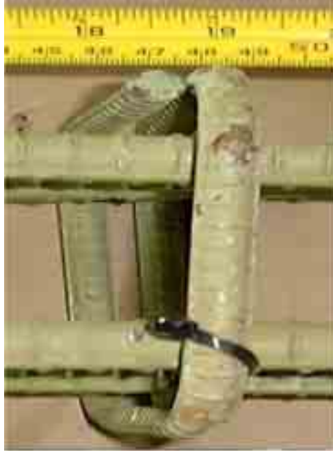
Figure 4.16: Observed Corrosion of Hoop in the Submerged Zone
