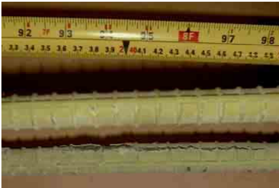
Figure 4.21: Disbondment of the Epoxy Coating in the Tidal Zone
