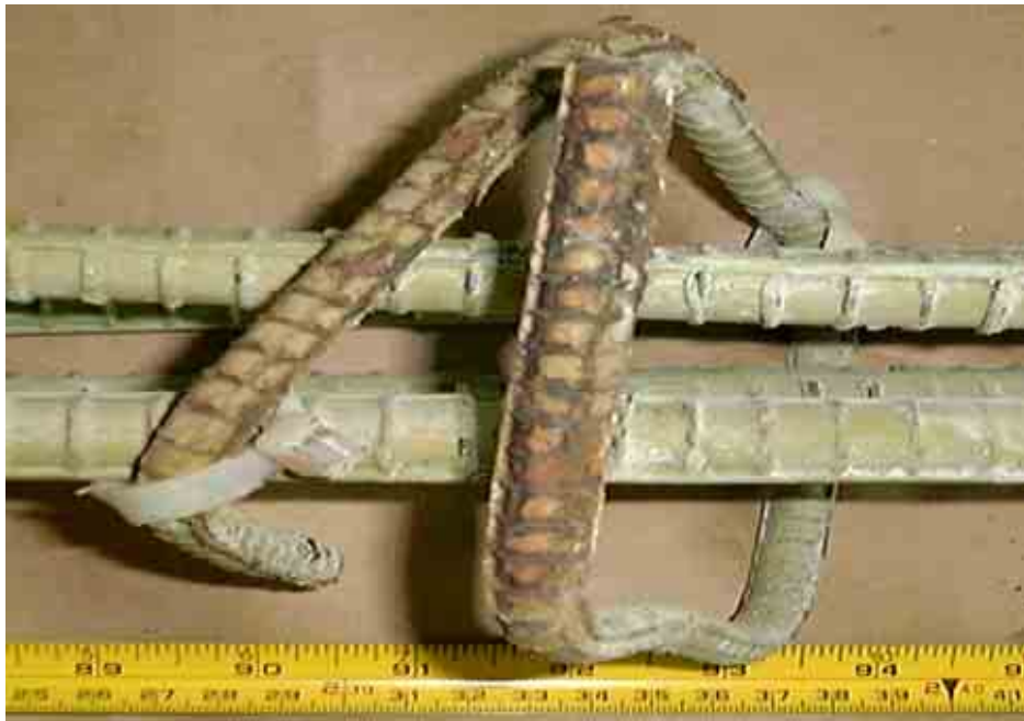
Figure 4.19: Hoop Corrosion in the Tidal Zone
