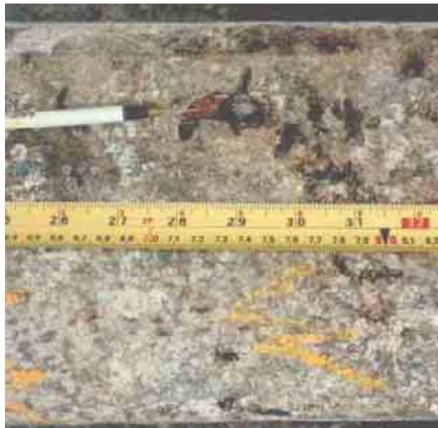
Figure 4.5: West Face of the Beam with Pockmarked Areas
