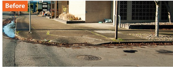
Above: A non-ADA-compliant sidewalk curb ramp on North Lombard Street before improvements.
