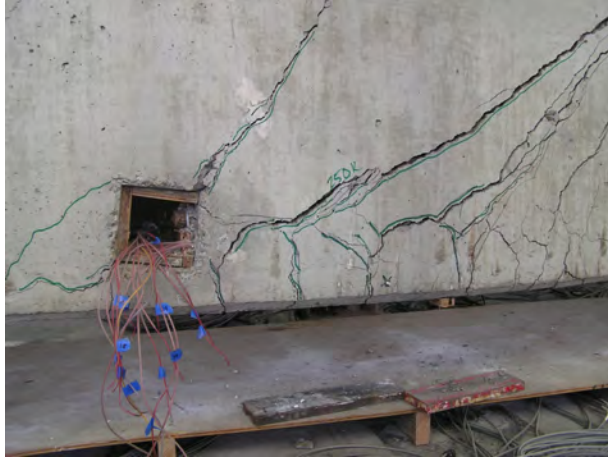
Figure C.2: Horizontal cracking along developing length of cutoff reinforcement in T specimen
