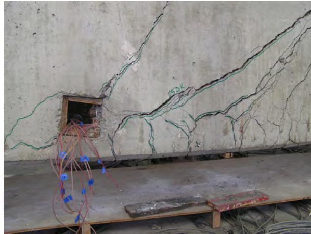
Figure 4.7: Typical anchorage cracking caused by slip of the cutoff bars in T-beam specimens
