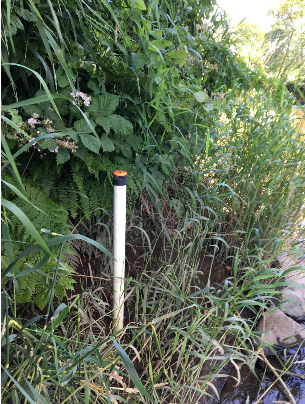
Figure 3.8: Photograph of the second installation of the Salmon River at Lincoln County Bridge station. The photograph is taken looking upstream, and the bridge pier is out of frame to the upper left. Photograph taken looking upstream, facing east.
