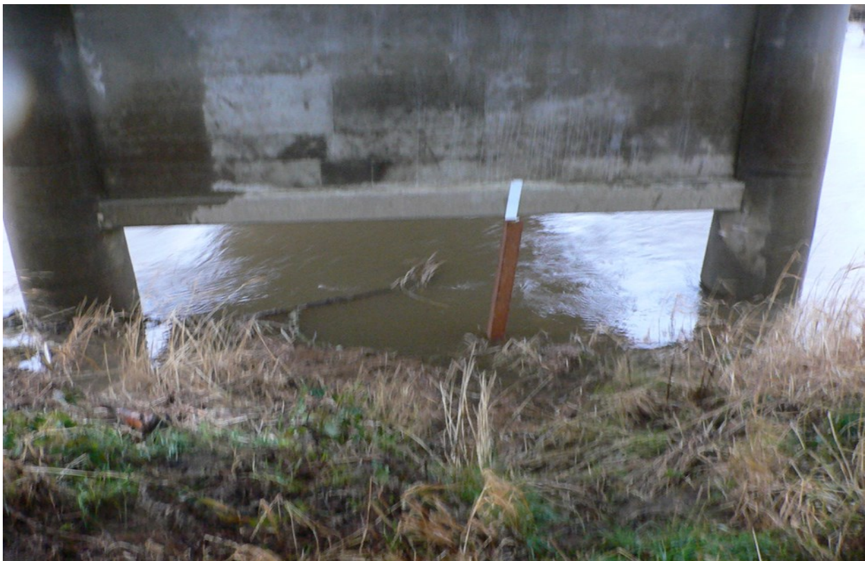
Figure 3.6: Photograph showing the original Lincoln County bridge station. Photograph taken facing southwest.
