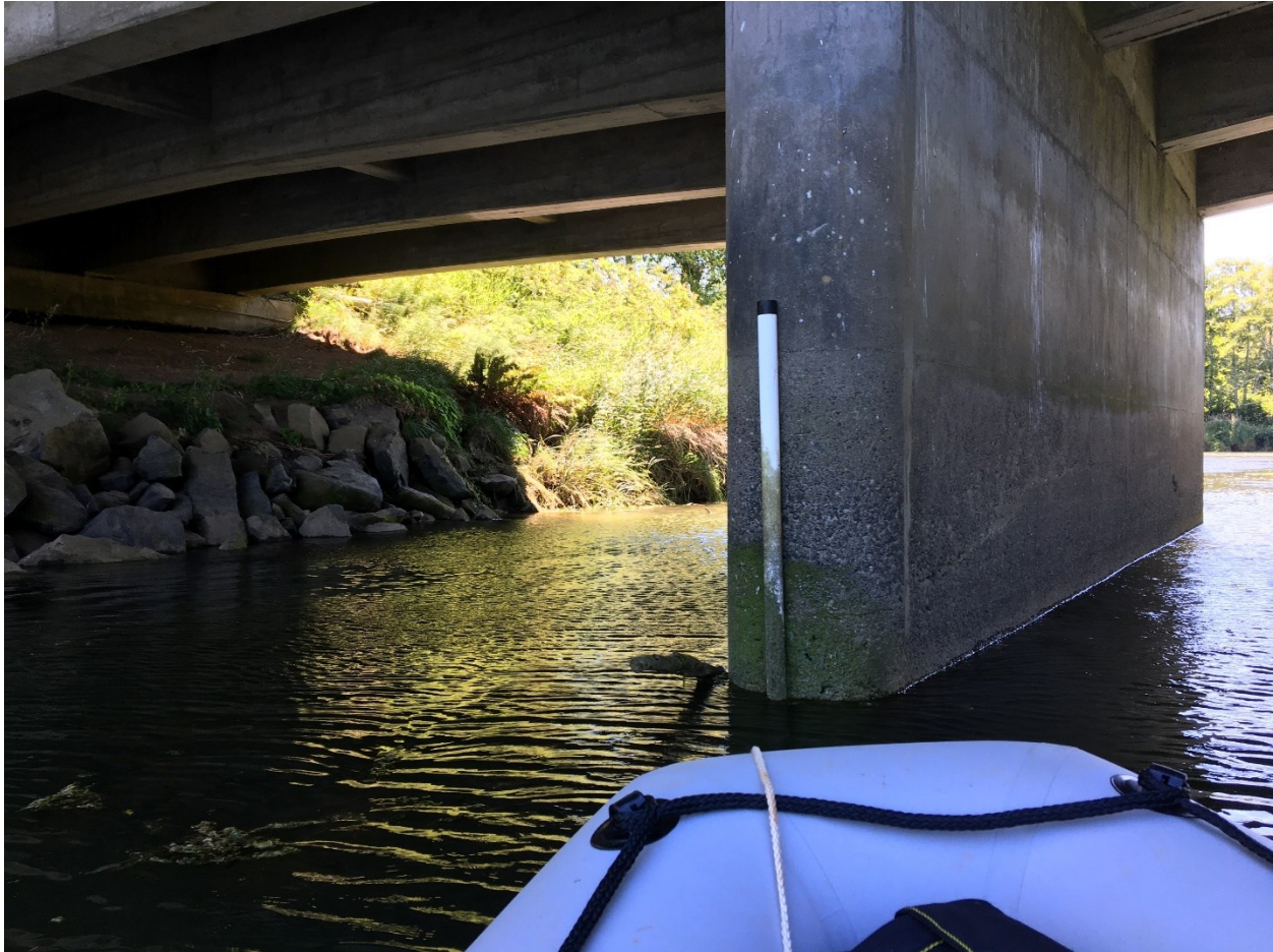
Figure 3.5: Photograph of the station installed on the bridge that carries US Route 101 over Salmon River. The photograph was taken looking upstream, facing southeast.
