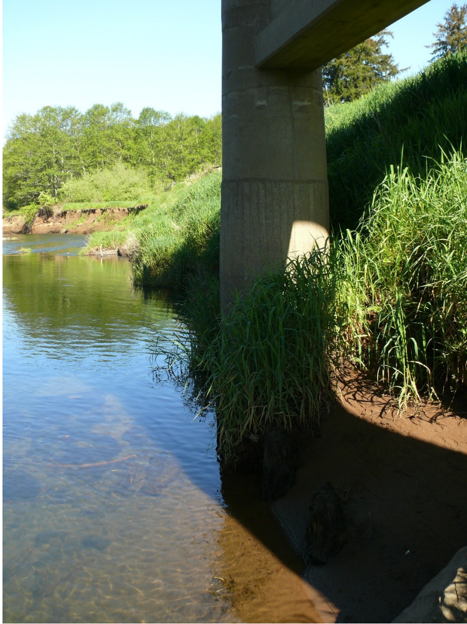
Figure 3.7: Photograph of Salmon River at Lincoln County bridge station location prior to installation. Photograph taken looking downstream, facing west.
