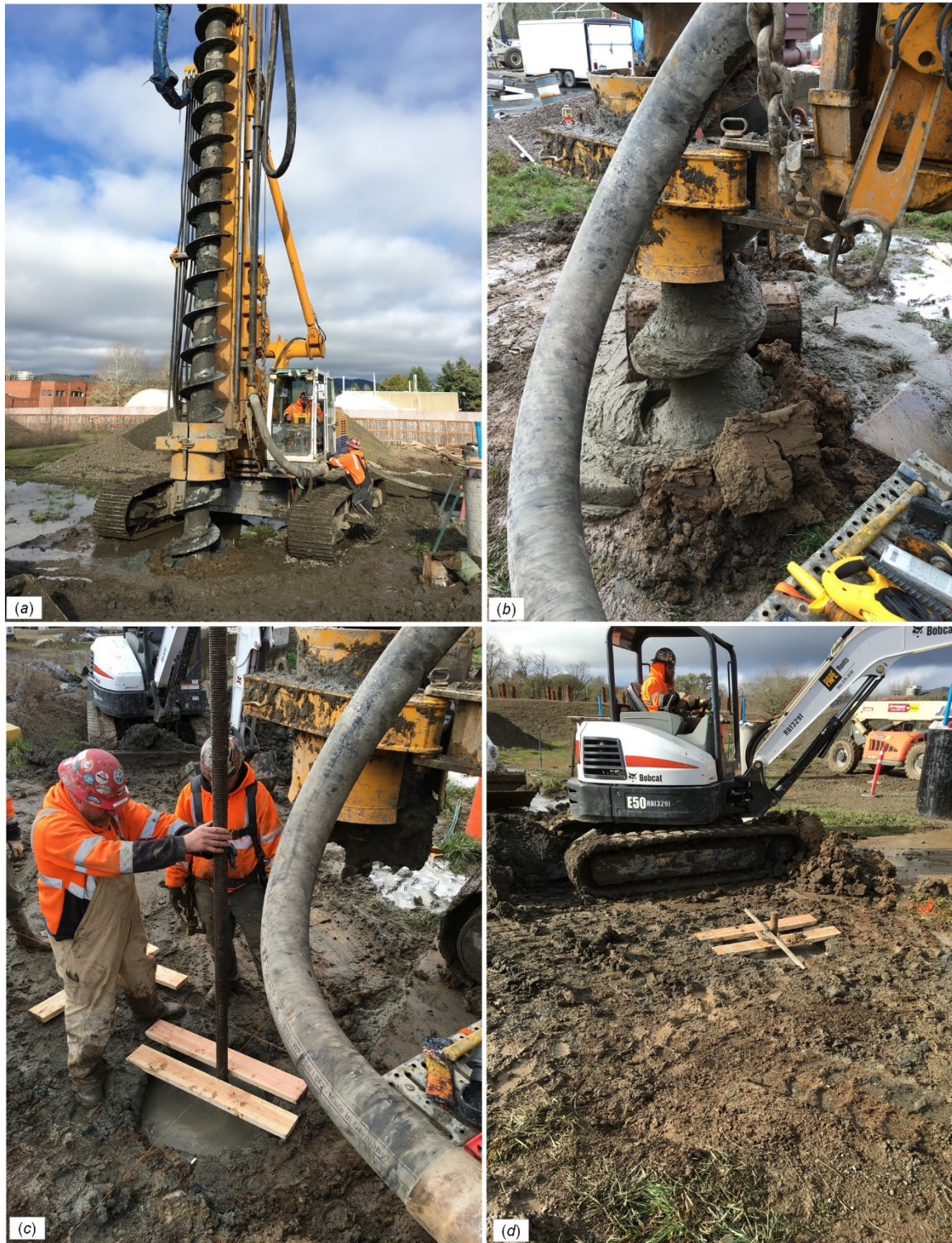
Figure 5.5: Construction of the continuous flight auger piles: (a) drilling a hole, (b) simultaneously pumping of the concrete and withdrawing of the auger, (c) lowering the steel bar, and (d) supporting the steel bar.
