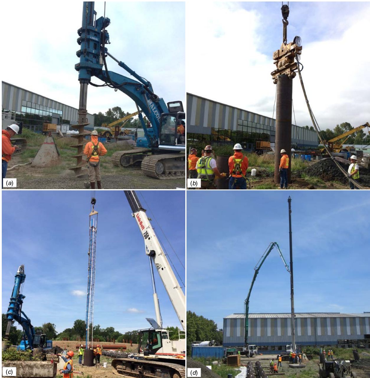
Figure 5.4: Construction of the cased shafts: (a) drilling a hole, (b) vibrating steel casing into the hole, (c) lowering the steel cage for CNIR, and (d) placing the concrete.
