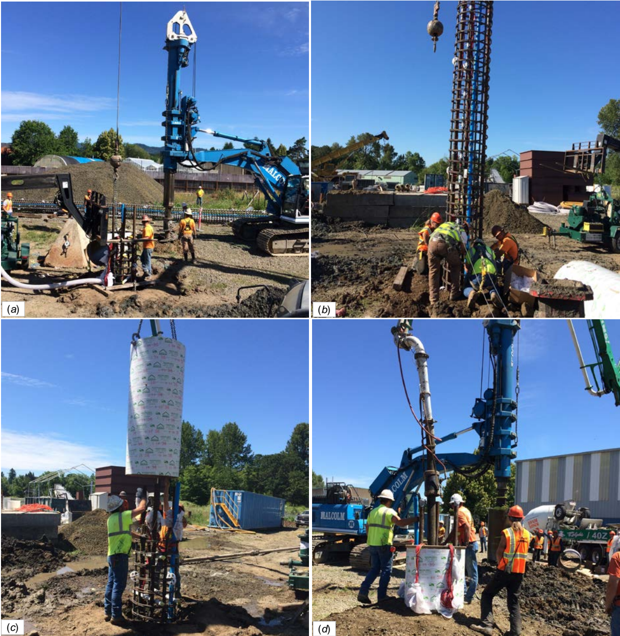
Figure 5.3: Construction of the uncased shafts: (a) drilling a hole, (b) lowering the steel cage into the hole, (c) installing sonotube concrete form, and (d) placing the concrete.
