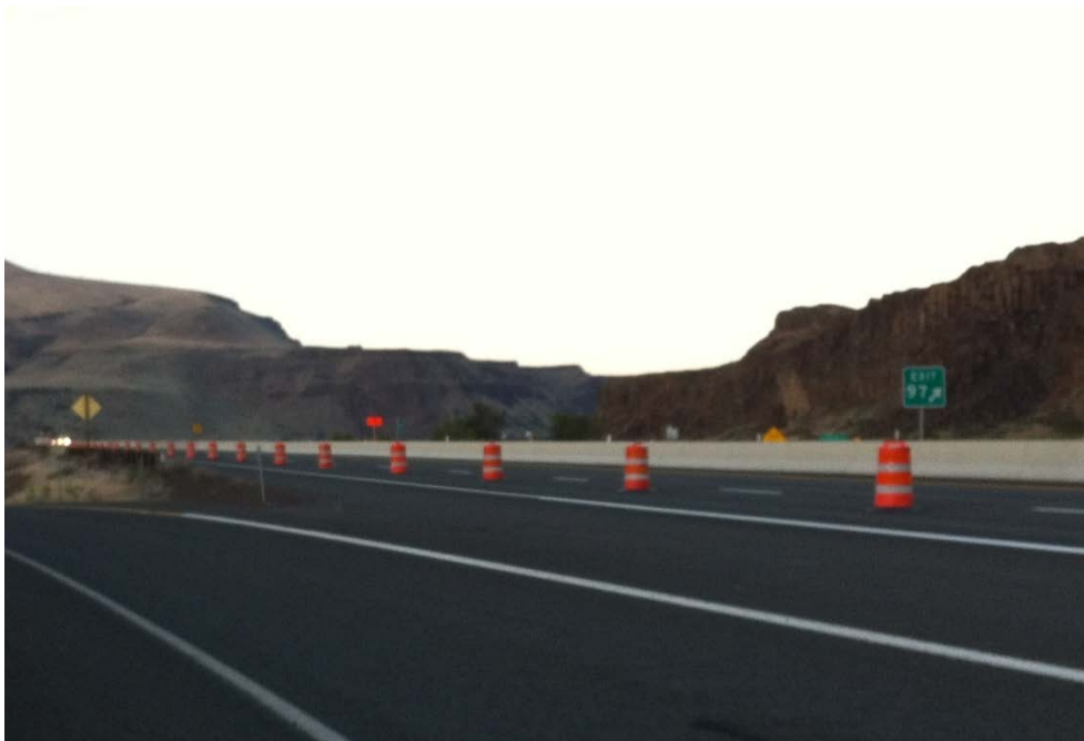
Figure 2.3: Plastic Drums on Roadway
