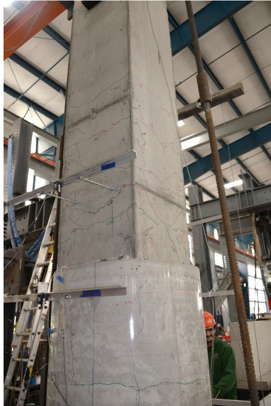
Figure 4.29: Specimen RS-T-R-LTi-90: Flexural and diagonal cracking above shell
