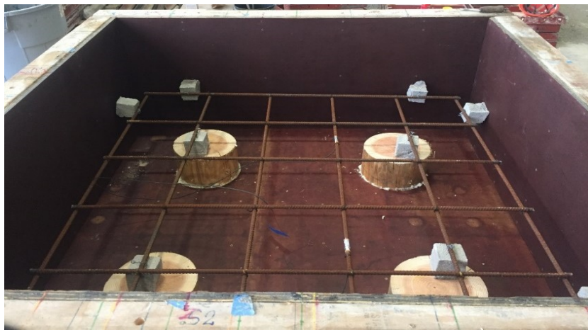
Figure 3.30: Image of timber pile cap prior to placement of column starter bars and casting concrete
