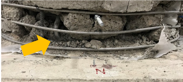
Figure 4.9: Specimen R-S-R-LTi-135: Buckled and fractured NE TiAB ligament at the bottom of the retrofit shell due to column sliding
