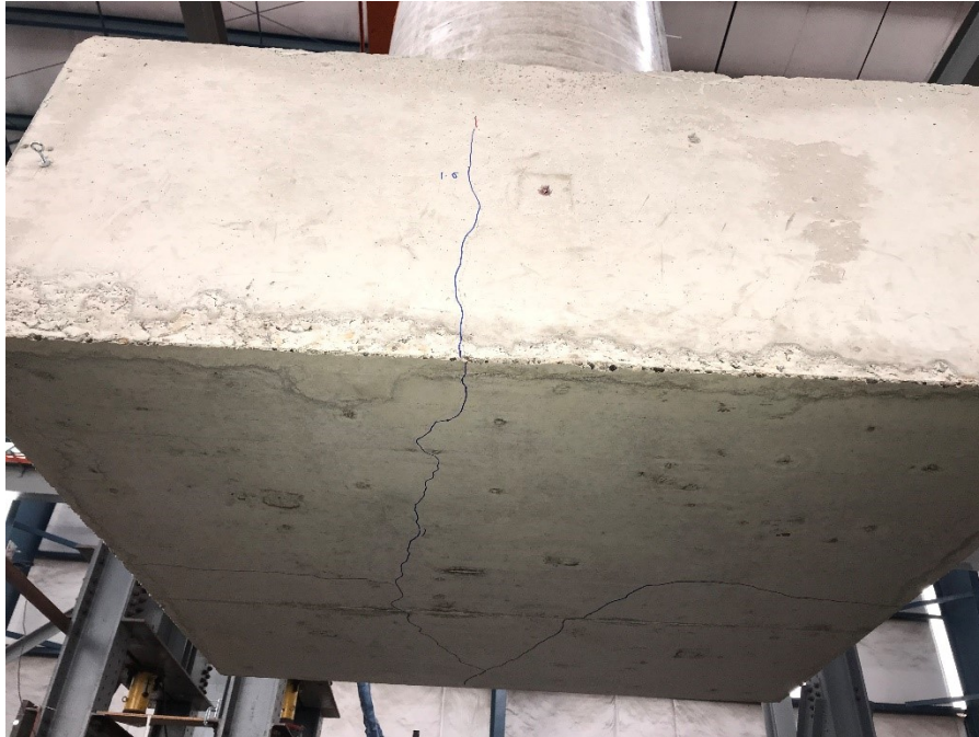
Figure 4.20: Specimen R-S-R-LTi-90-Spread: Cracking on spread footing
