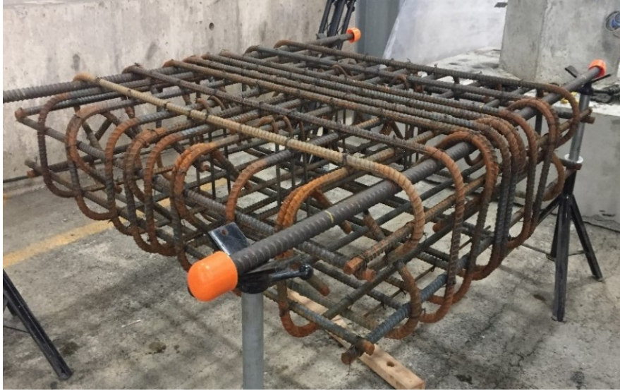
Figure 3.25: Photograph of typical footing reinforcing details (not typical of footing designs for vintage columns)
