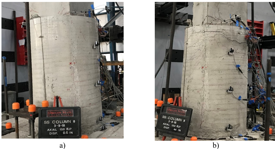
Figure 4.16: Specimen R-S-R-LSS-90: Progression of visual distress: a) at 0.6 in (approx. 0.6%) drift level, b) at 4.4 in drift (approx. 4.4%) drift level
