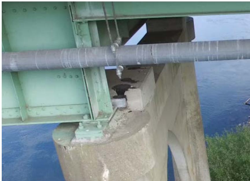
Figure 3.11: Example photo taken with a visible-spectrum camera on a UAS of a bridge steel-to-concrete bearing connection; note the possible leaking joint at this connection
