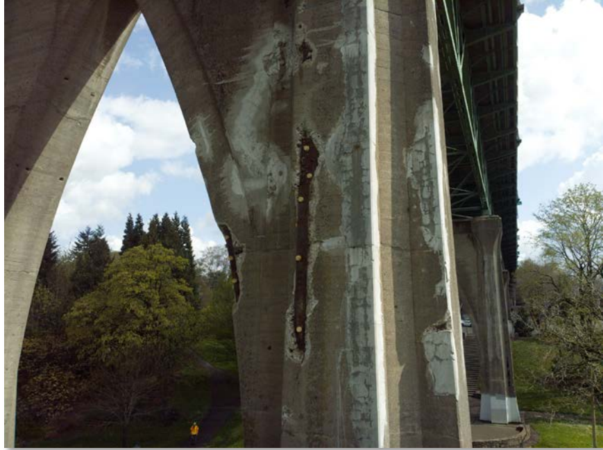
Figure 4.58: Spalling with exposed metal on bent 11. Taken from senseFly albris main HD camera. Focal length: 8 mm, 35mm equivalent: 25 mm. (Full image)
