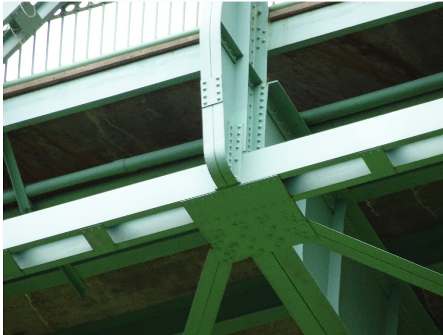
Figure 4.29: Photo of northeast connection on span 6. Taken from S900 equipped with a Sony DSC-WX500 optical zoom digital camera. Focal length: 85 mm, 35mm; equivalent: 500 mm
