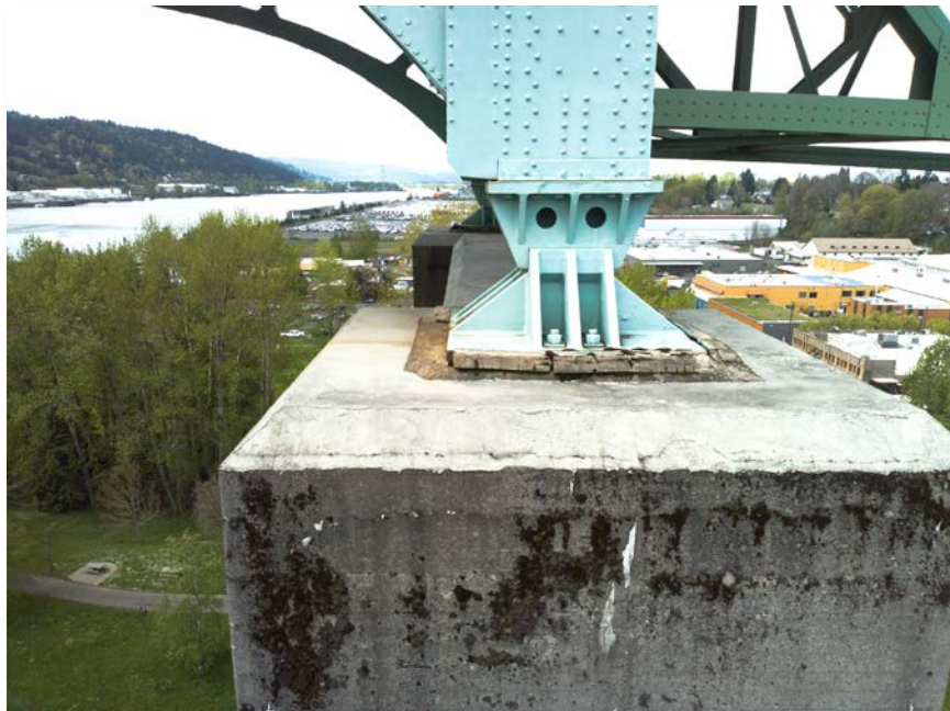
Figure 4.67: South bearing pad connection on top of bent 7. Taken from senseFly albris main HD camera. Focal length: 8 mm, 35mm equivalent: 25 mm. (Full image)
