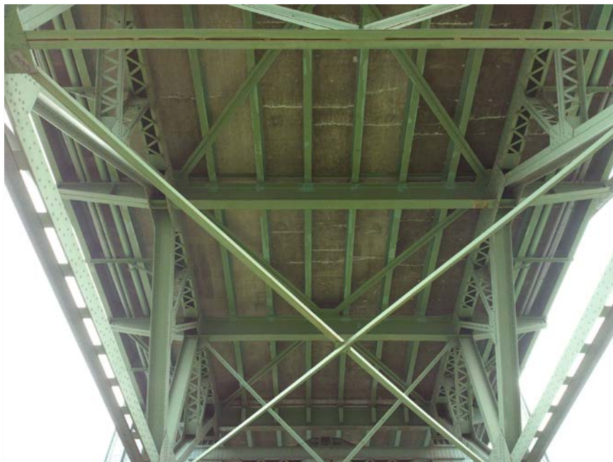
Figure 4.69: Cross bracing and traverse cracking with efflorescence in deck soffit in span 7. Taken from senseFly albris main HD camera. Focal length: 8 mm, 35mm equivalent: 25 mm. (Full image)
