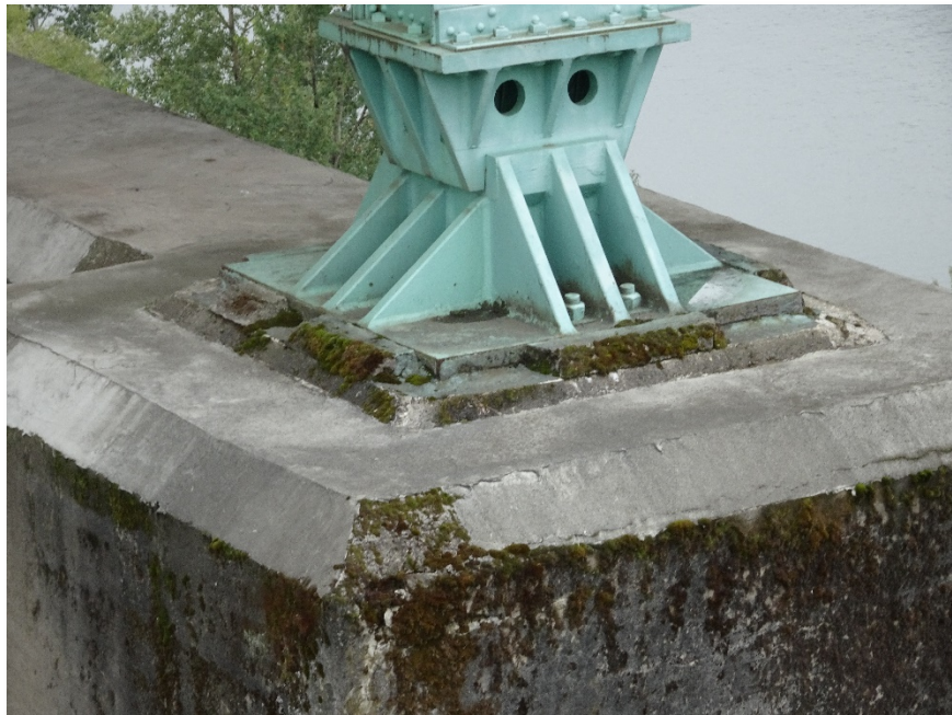
Figure 4.35: Bearing pad connection on the top north side of Bent 7. Taken from S900 equipped with a Sony DSC-WX500 optical zoom digital camera. Focal length: 24 mm, 35mm equivalent: 139 mm. (Full image)
