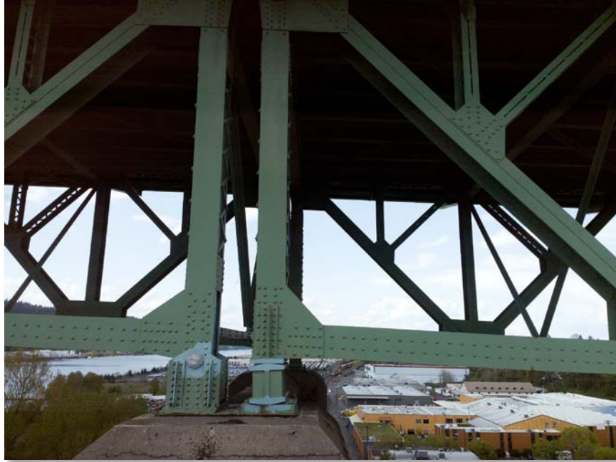
Figure 4.64: South pin connection on top of bent 8. Taken from senseFly albris main HD camera. Focal length: 8 mm, 35mm equivalent: 25 mm. (Full image)
