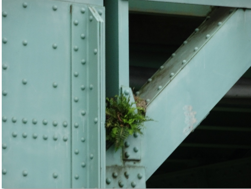
Figure 4.38: Vegetation growing on northeast side of span 6. Taken from S900 equipped with a Sony DSC-WX500 optical zoom digital camera. Focal length: 54 mm, 35mm equivalent: 316 mm. (Full image)
