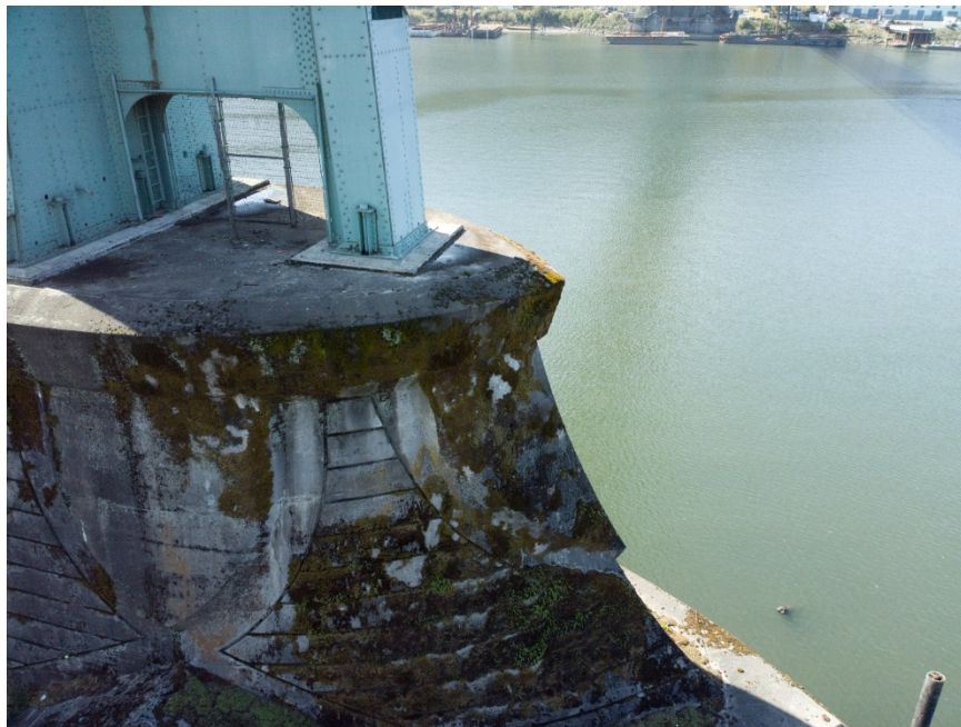
Figure 4.47: North side of the East tower footing. Taken from senseFly albris main HD camera. Focal length: 8 mm, 35mm equivalent: 25 mm. (Full image)
