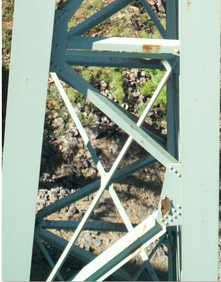
Figure 4.26: Northern support tower of the bridge with large areas of rust and peeled paint on members and gusset plates. (Cropped image)
