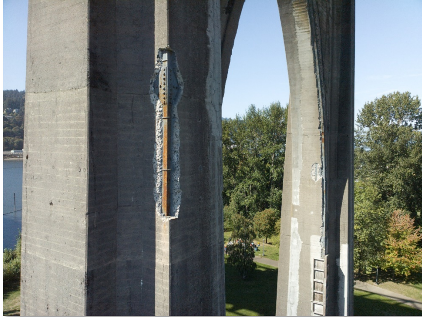
Figure 4.48: Significant spalling with exposed metal on bent 7. Taken from senseFly albris main HD camera. Focal length: 8 mm, 35mm equivalent: 25 mm. (Full image)
