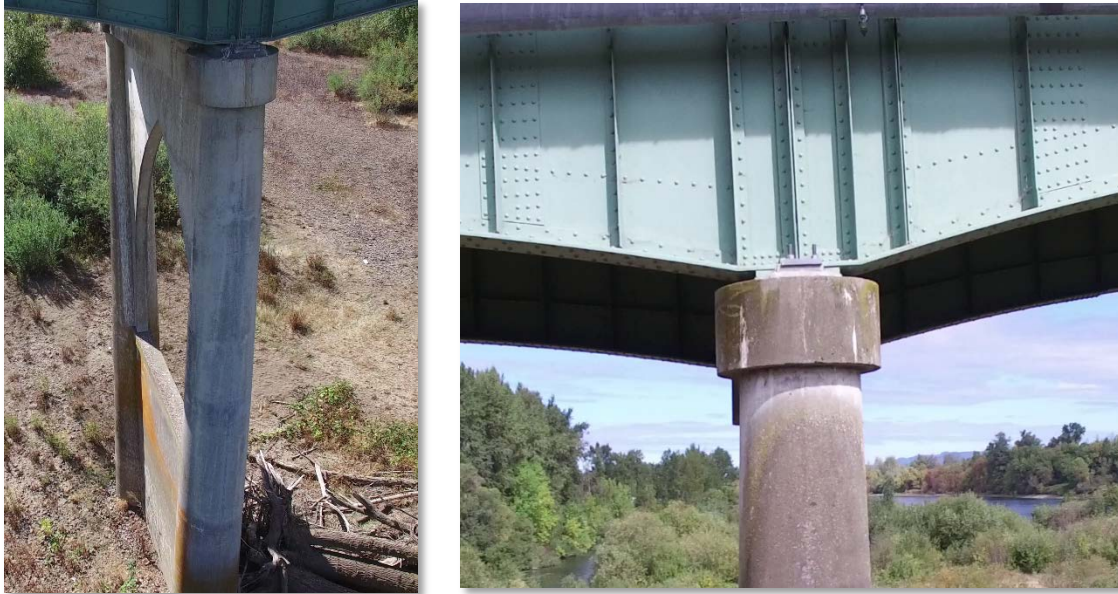
Figure 4.8: Efflorescence on concrete columns. (Cropped images)
