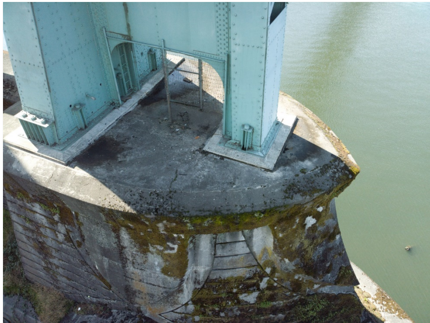
Figure 4.43: North side of the East tower footing. Taken from senseFly albris main HD camera. Focal length: 8 mm, 35mm equivalent: 25 mm. (Full image)
