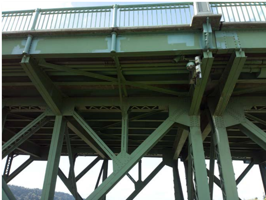
Figure 4.63: Under the south east soffit of span 8. Note the areas where the paint has been refinished is very noticeable. Taken from senseFly albris main HD camera. Focal length: 8 mm, 35mm equivalent: 25 mm. (Full image)
