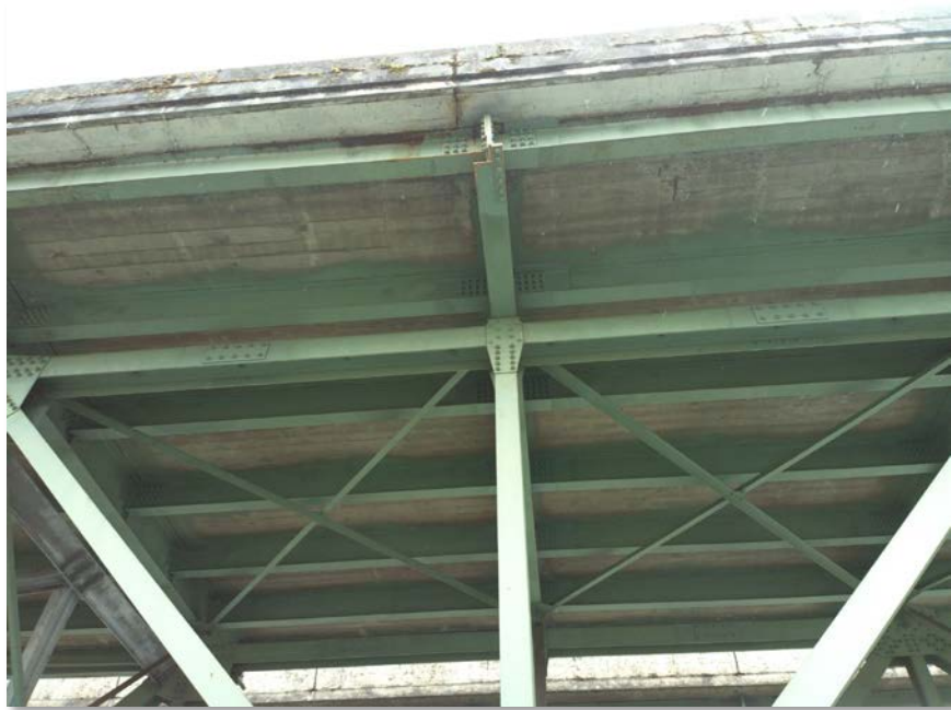
Figure 4.55: Spalling with exposed rebar in deck soffit. Taken from senseFly albris main HD camera. Focal length: 8 mm, 35mm equivalent: 25 mm. (Full image)
