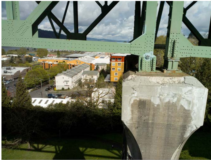
Figure 4.57: South pin connection on top of bent 11. Taken from senseFly albris main HD camera. Focal length: 8 mm, 35mm equivalent: 25 mm. (Full image)
