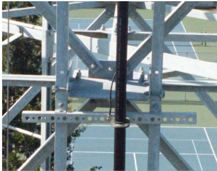
Figure 4.108: Communication cable mount on the Corvallis Maintenance Tower
