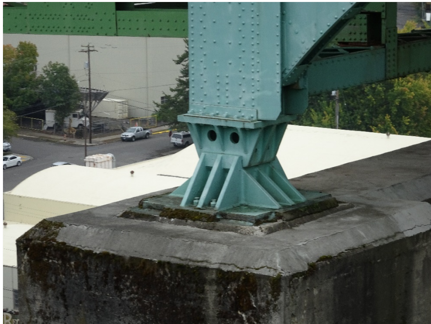
Figure 4.31: Bearing pad connection on the top north side of Bent 7. Taken from S900 equipped with a Sony DSC-WX500 optical zoom digital camera. Focal length: 26 mm, 35mm equivalent: 154 mm
