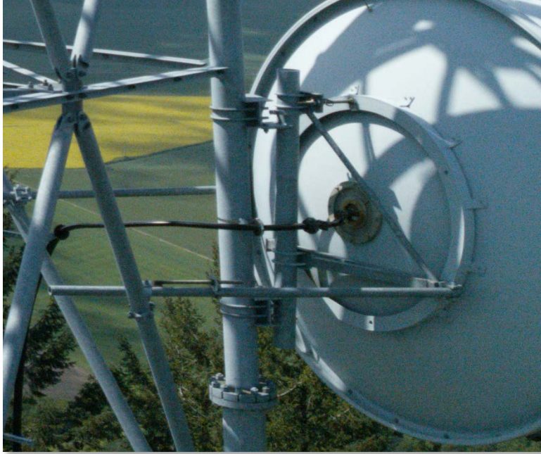
Figure 4.98: Antenna connection at the Washburn Butte Tower
