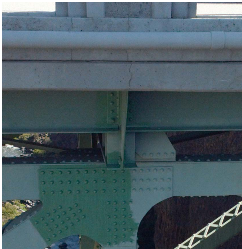
Figure 4.15: Deck bearing girder connection on Crooked River Bridge. Note the small crack in the deck at the location of support and recent paint patchwork in darker green. (Cropped image)
