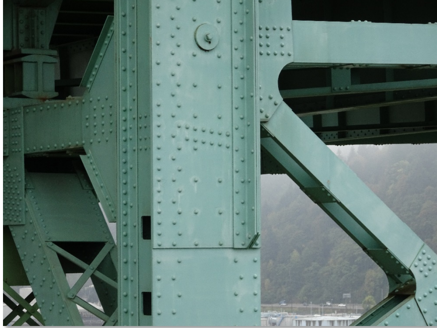
Figure 4.36: Large bolt on the northeast side of span 6. Taken from S900 equipped with a Sony DSC-WX500 optical zoom digital camera. Focal length: 24 mm, 35mm equivalent: 139 mm. (Full image)
