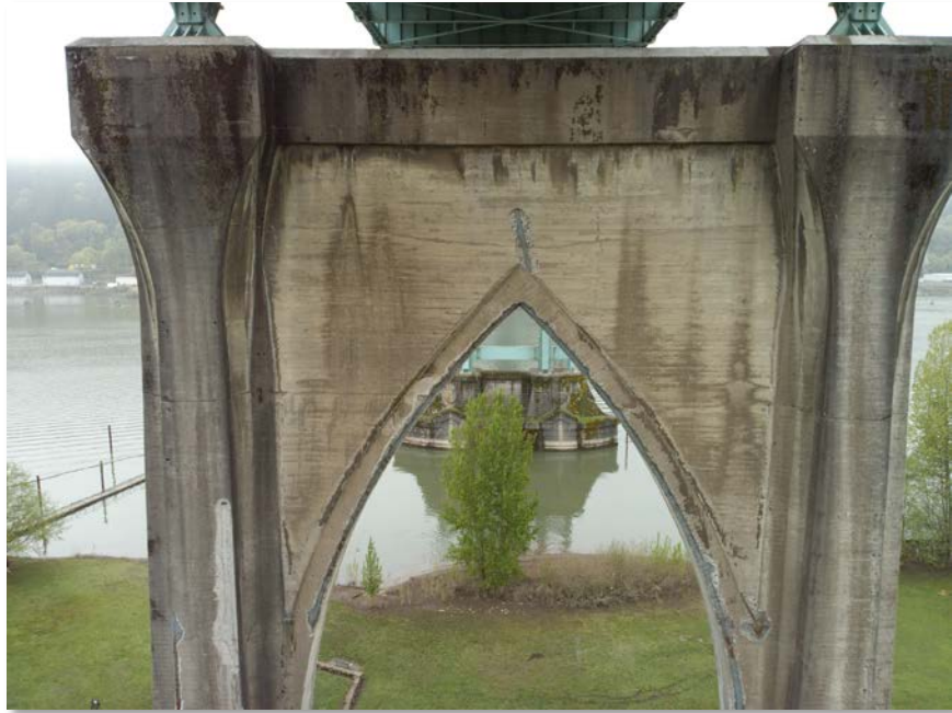
Figure 4.70: Top east side of bent 7 showing spalling with exposed metal at the top of the arch. Taken from senseFly albris main HD camera. Focal length: 8 mm, 35mm equivalent: 25 mm. (Full image)
