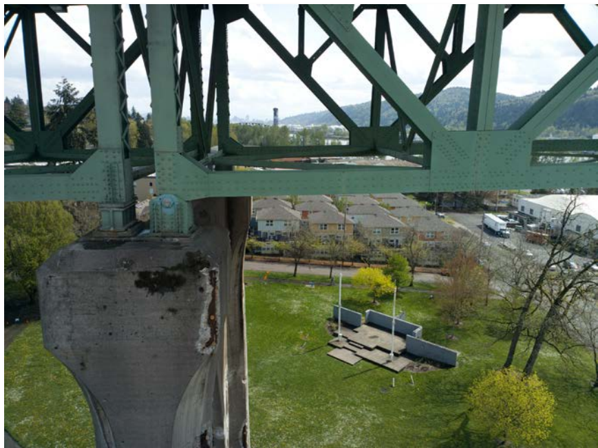
Figure 4.61: North pin connection on top of bent 11. Taken from senseFly albris main HD camera. Focal length: 8 mm, 35mm equivalent: 25 mm. (Full image)
