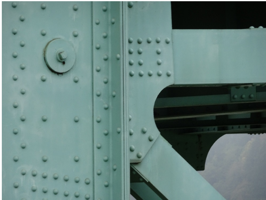
Figure 4.37: Large bolt on the northeast side of span 6. Taken from S900 equipped with a Sony DSC-WX500 optical zoom digital camera. Focal length: 54 mm, 35mm equivalent: 316 mm. (Full image)
