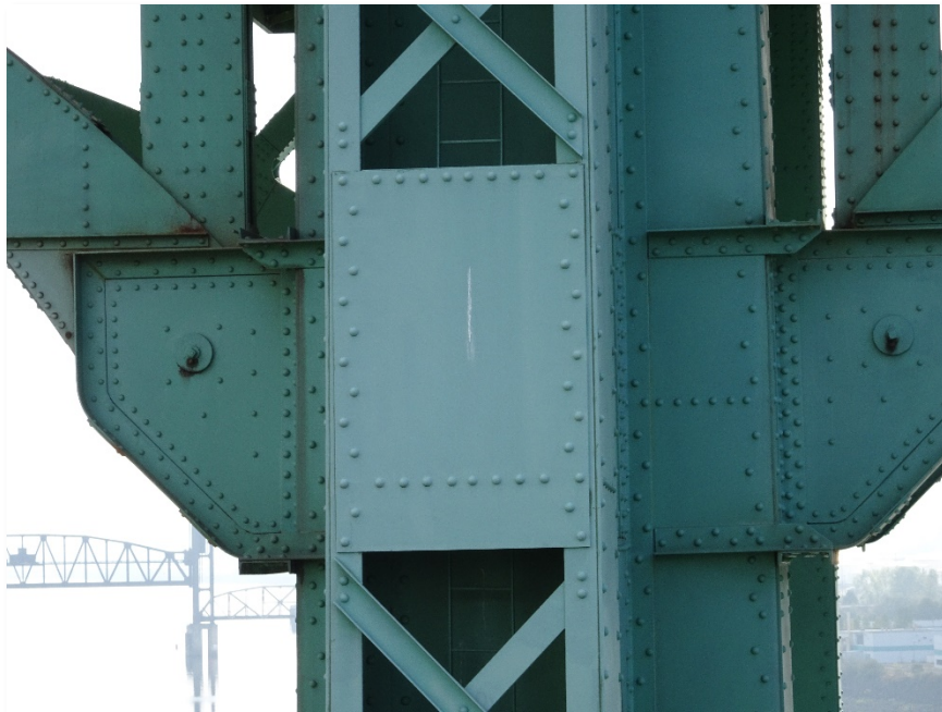
Figure 4.39: Large bolt connection for lower cord of spans 5 (right) and 6 (left) on North side of east tower. Taken from S900 equipped with a Sony DSC-WX500 optical zoom digital camera. Focal length: 21 mm, 35mm equivalent: 123 mm. (Full image)
