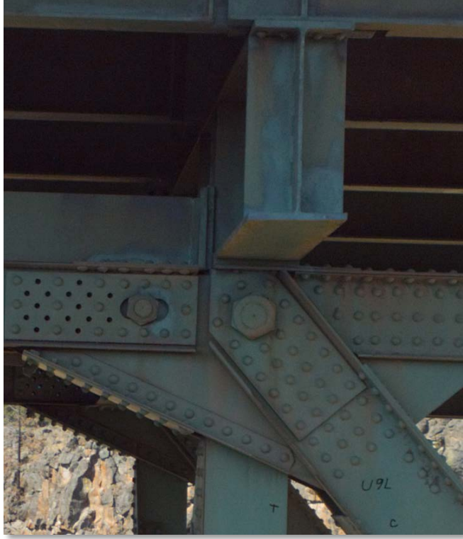
Figure 4.24: Mid span connection pin at upper chord of Mill Creek Bridge. Note that lettering written by inspectors during previous inspections are legible in the image. (Cropped image)
