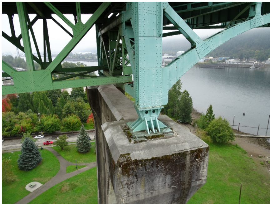
Figure 4.33: Bearing pad connection on the top north side of Bent 7. Taken from S900 equipped with a Sony DSC-WX500 optical zoom digital camera. Focal length: 4 mm, 35mm equivalent: 24 mm. (Full image)
