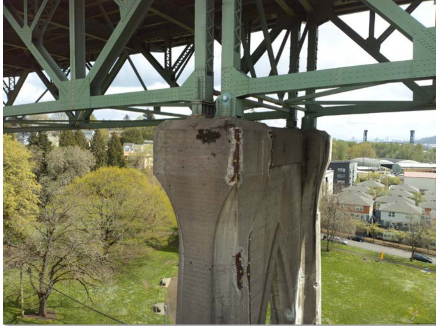
Figure 4.62: Spalling on top of the north side of bent 11 with exposed metal. Taken from senseFly albris main HD camera. Focal length: 8 mm, 35mm equivalent: 25 mm. (Full image)
