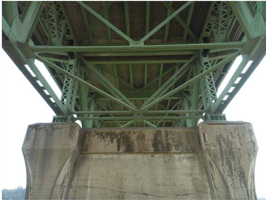
Figure 4.65: Top east side of bent 8. Taken from senseFly albris main HD camera. Focal length: 8 mm, 35mm equivalent: 25 mm. (Full image)
