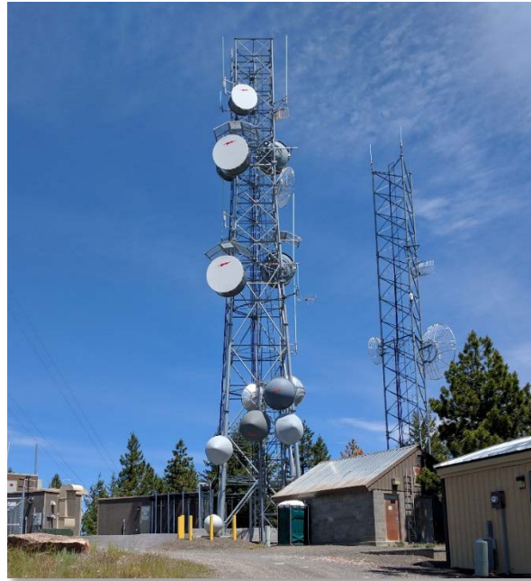
Figure 4.109: Grizzly Mountain Communication Towers
