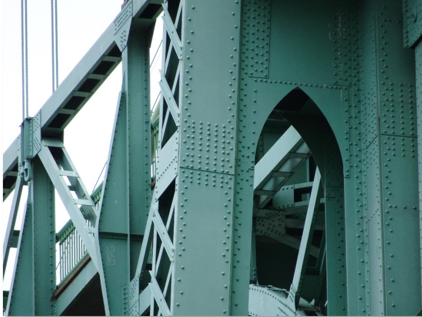
Figure 4.30: Northwest side of east tower (bent 6). Taken from S900 equipped with a Sony DSC-WX500 optical zoom digital camera. Focal length: 123 mm, 35mm equivalent: 700 mm
