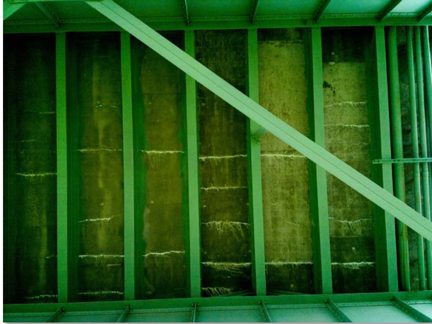
Figure 4.68: Traverse cracking with efflorescence in deck soffit at southeast end of span 6. Taken from senseFly albris main HD camera. Focal length: 8 mm, 35mm equivalent: 25 mm. (Full image)
