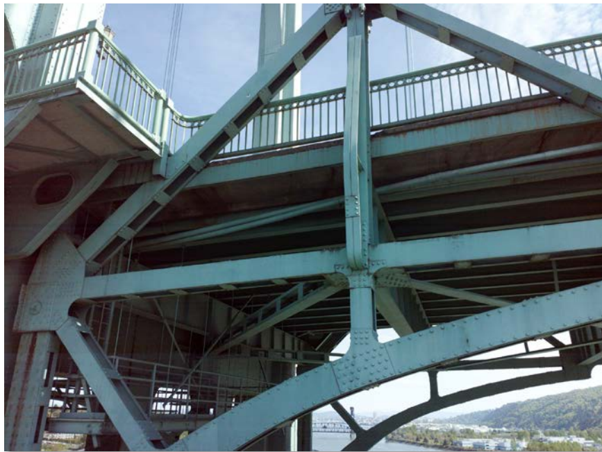
Figure 4.83: Looking under the deck at the northwest connection of span 5 to the east tower. Taken from senseFly albris main HD camera. Focal length: 8 mm, 35mm equivalent: 25 mm. (Full image)
