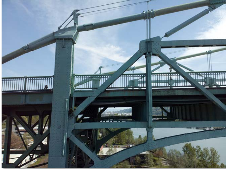
Figure 4.82: North east side of span 6 connection at bent 7. Taken from senseFly albris main HD camera. Focal length: 8 mm, 35mm equivalent: 25 mm. (Full image)
