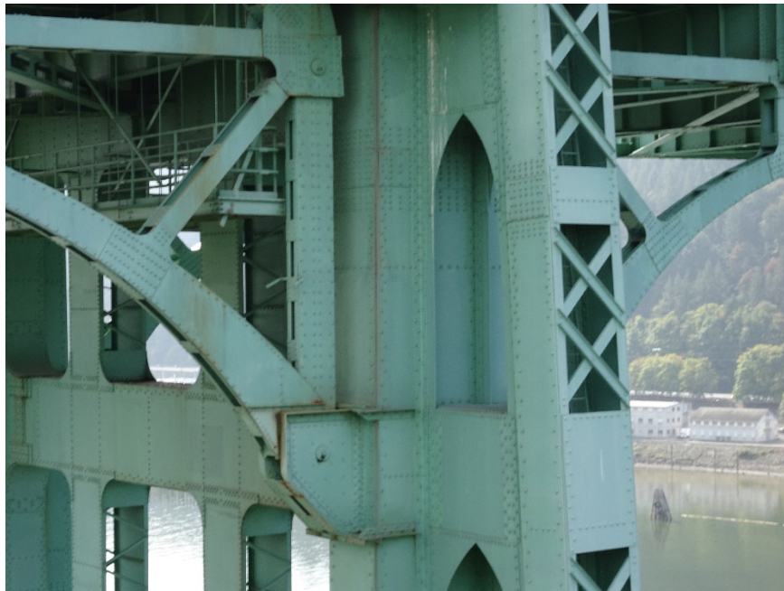
Figure 4.41: Connection for span 6 (left) to North side of east tower. Taken from S900 equipped with a Sony DSC-WX500 optical zoom digital camera. Focal length: 13 mm, 35mm equivalent: 75 mm. (Full image)
