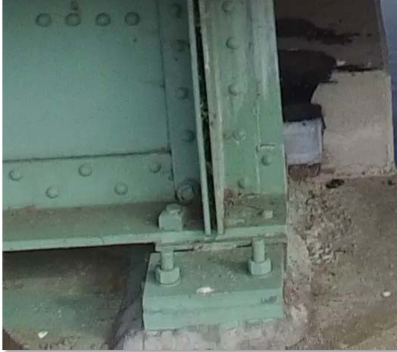
Figure 4.6: Connection of steel member to concrete tower; note the missing bolt nut. (Cropped image)
