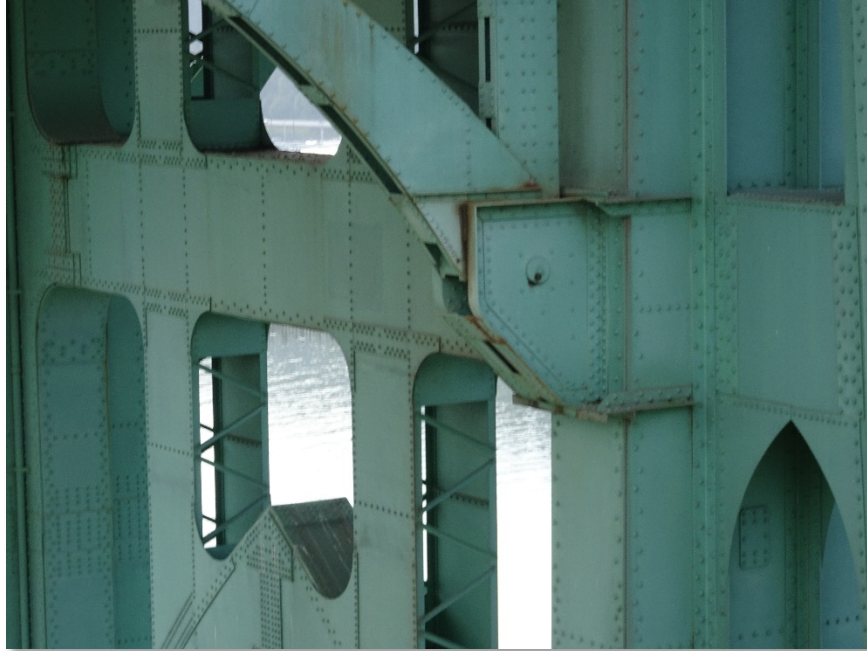
Figure 4.42: Large bolt connection for lower cord of spans 6 left on North side of east tower. Taken from S900 equipped with a Sony DSC-WX500 optical zoom digital camera. Focal length: 19 mm, 35mm equivalent: 112 mm. (Full image)
