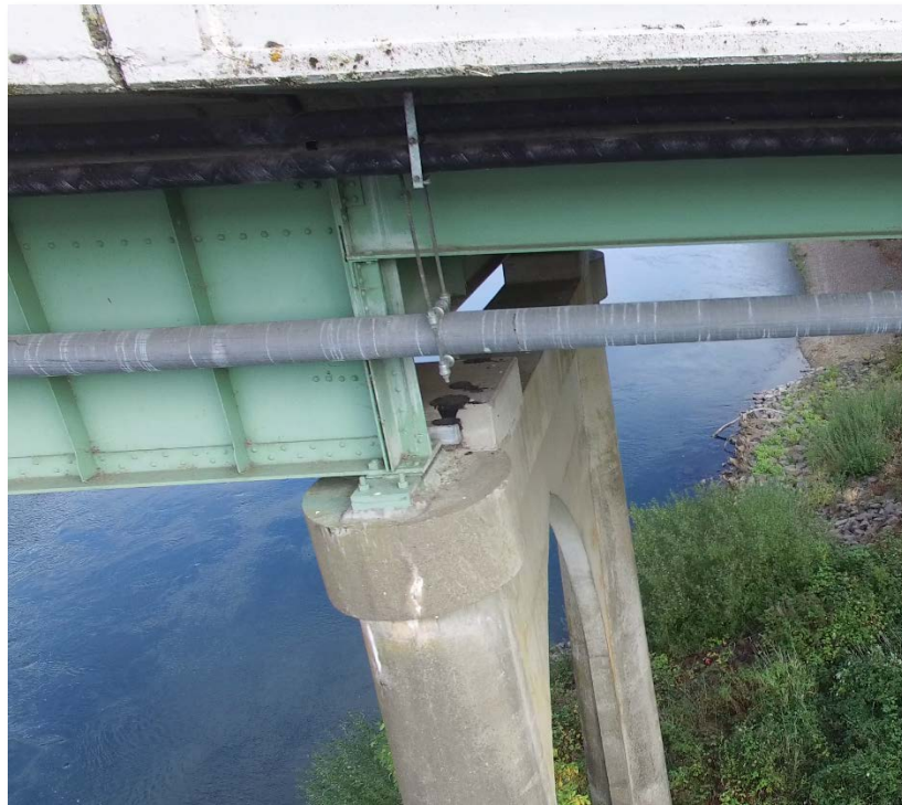
Figure 4.3: Evidence of a leaking joint. (Cropped image)
