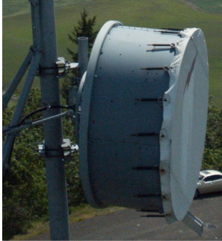
Figure 4.96: Antenna and its connection at the Washburn Butte Tower
