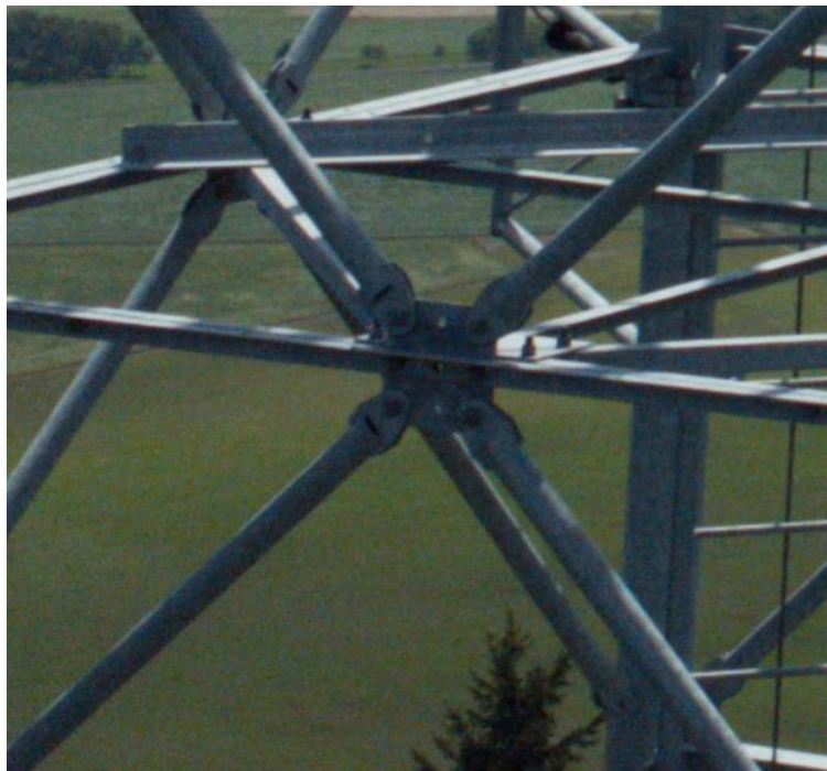
Figure 4.97: Member cross bracing connection at the Washburn Butte Tower. Notice it is possible to identify missing bolts at this connection
