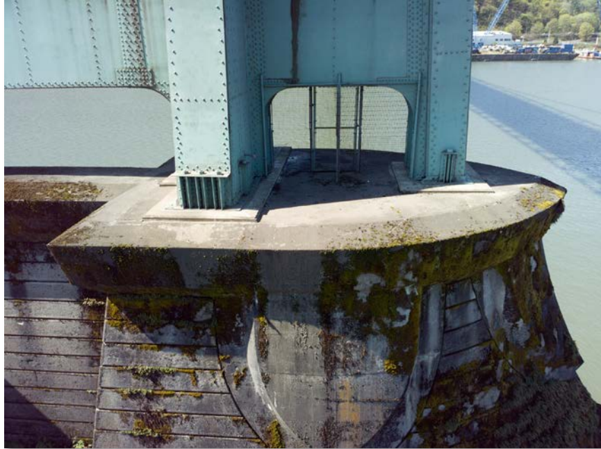
Figure 4.74: North side of the East tower footing. Taken from senseFly albris main HD camera. Focal length: 8 mm, 35mm equivalent: 25 mm. (Full image)
