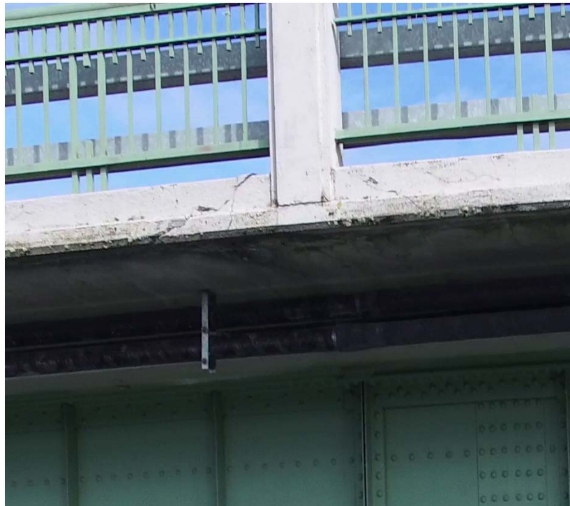
Figure 4.5: Cracking of concrete railing. (Cropped image)
