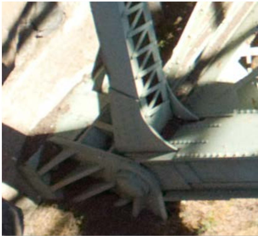
Figure 4.19: Lower abutment connection on northwest corner of bridge - into the wall of the gorge. Note the shadow at this location (Cropped image)
