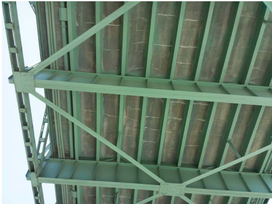
Figure 4.77: Looking under span 5. Taken from senseFly albris main HD camera. Focal length: 8 mm, 35mm equivalent: 25 mm. (Full image)
