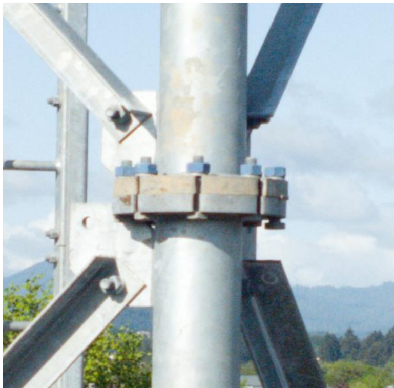
Figure 4.106: Loose bolt on northwest column of the Corvallis Maintenance Tower. (Note ODOT loosened this bolt as a blind test on if it could be detected during a UAS inspection.)
