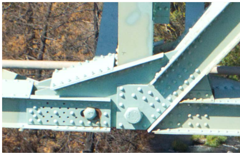
Figure 4.27: One of the lower chord connection plates on the bridge. Note the rust around the connection pin. (Cropped image)
