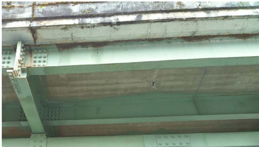
Figure 4.52: Spalling with exposed rebar in deck soffit. Taken from senseFly albris main HD camera. Focal length: 8 mm, 35mm equivalent: 25 mm. (Cropped image)
