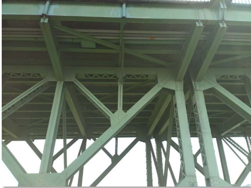
Figure 4.60: Looking under the North West side of span 10. Note the conduit failure. Taken from senseFly albris main HD camera. Focal length: 8 mm, 35mm equivalent: 25 mm. (Full image)
