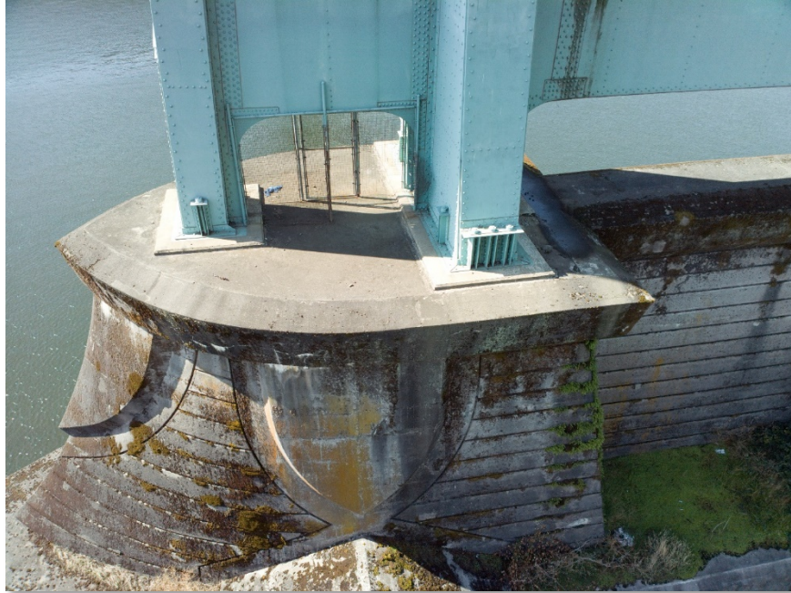
Figure 4.44: South side of the East tower footing. Taken from senseFly albris main HD camera. Focal length: 8 mm, 35mm equivalent: 25 mm. (Full image)
