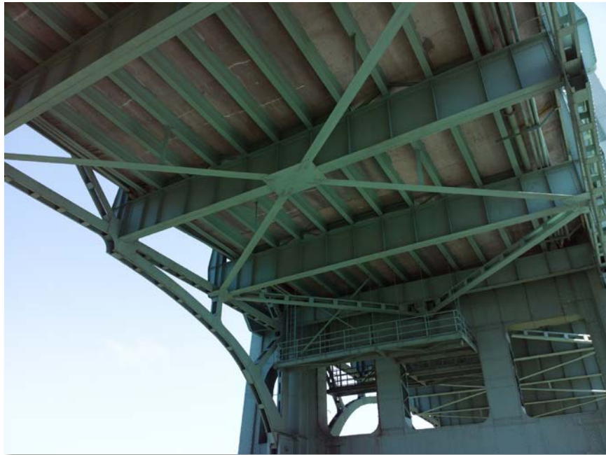
Figure 4.73: Looking under the deck at the northwest connection of span 5 to the east tower. Taken from senseFly albris main HD camera. Focal length: 8 mm, 35mm equivalent: 25 mm. (Full image)
