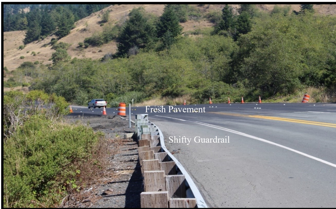
Figure 1.1: Evidence of damage to Highway 101 at the Hooskanaden Slide requiring routine repaving of the road (MP344, August 2016).
