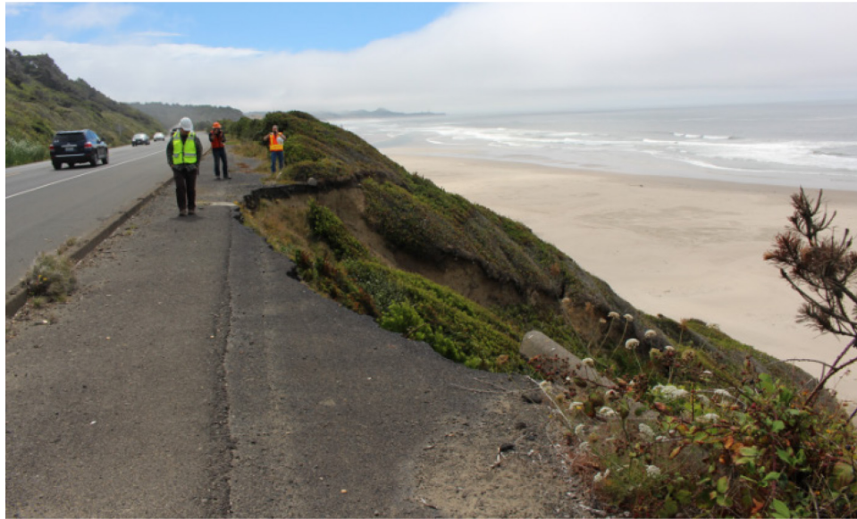
Figure 3.8: Mass movement and infrastructure damage along Highway 101 at Spencer Creek, (facing south, near MP 134, August 2016).
