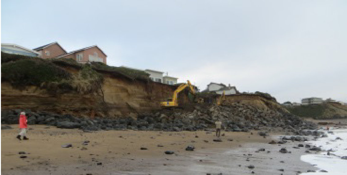
Figure 2.2: Sea cliff erosion located at Gleneden Beach, Lincoln County. The Photograph shows the presence of terrace sands that are rapidly eroding in response to cliff toe erosion. An emergency riprap structure is being constructed to mitigate the problem (Photo courtesy of J. Allan, DOGAMI, 2013).
