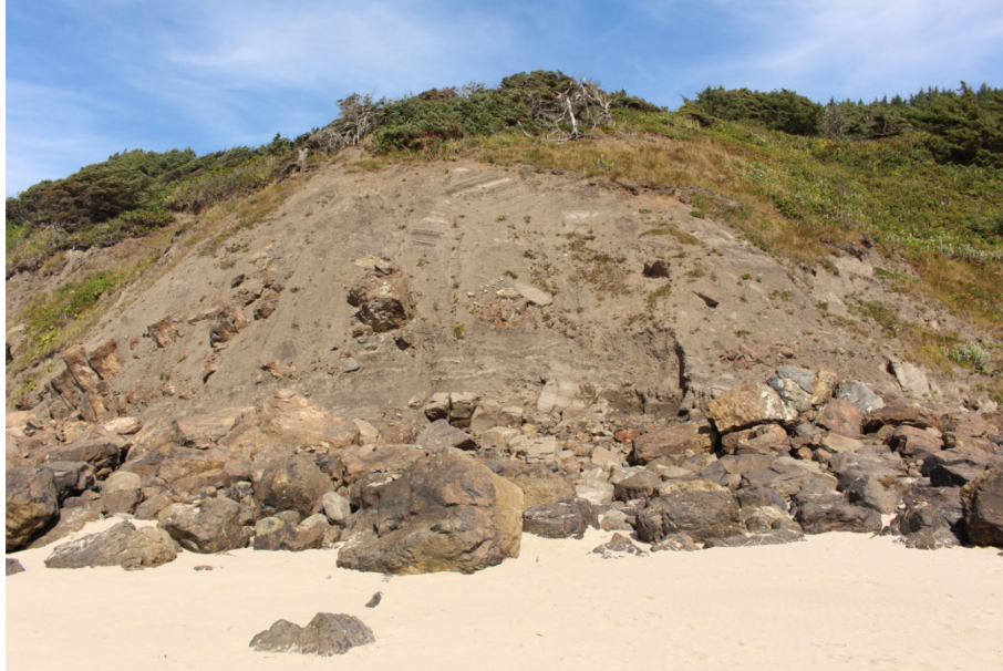
Figure 3.2: The coastal sea cliff at the most westerly point of Silver Point (facing east) (near MP32, August 2016).
