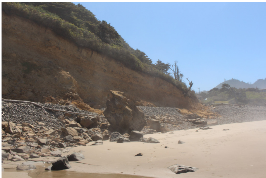
Figure 3.6: The coastal sea cliff and cobble/boulder berm along the toe of the Arch Cape site (facing southeast) (near MP36, August 2016).
