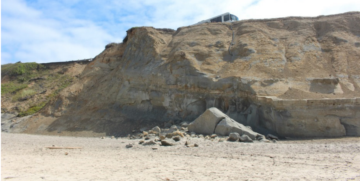
Figure 2.11: Recent sea cliff collapse at Beverly Beach near a broken drain pipe (near MP134, August 2016).
