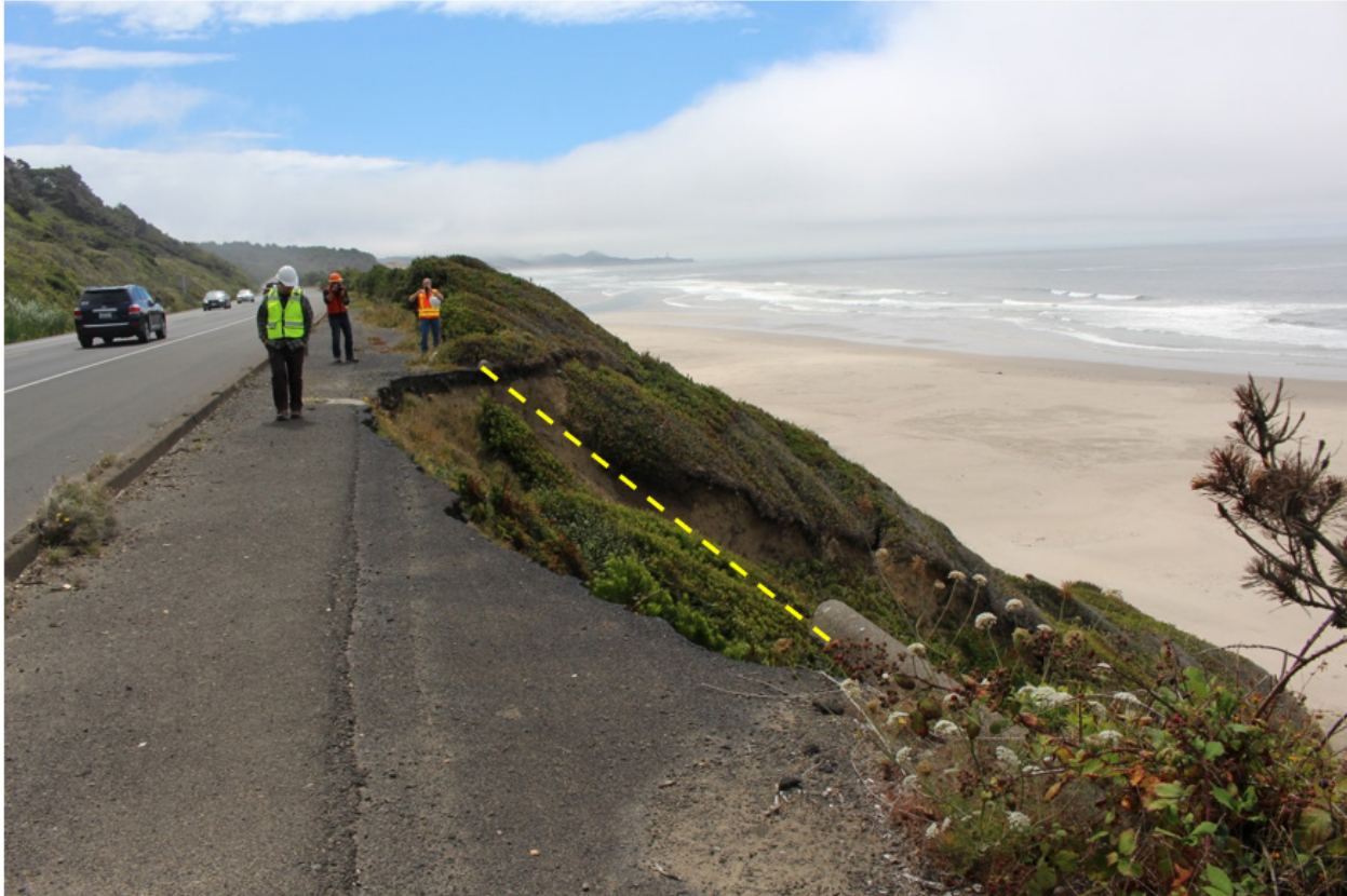
Figure 2.4: Sea cliff erosion occurring at Beverly Beach, OR. where Highway 101 runs parallel to the sea cliffs. In some cases, coastal landsliding and localized retrogression has resulted in relocation of the highway. The former location of a concrete curb is shown with the yellow, dashed line (near MP134, August 2016).
