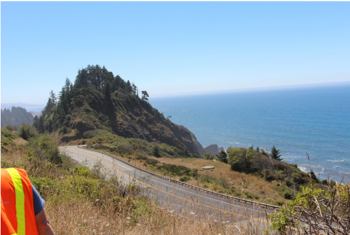
Figure 3.10: Photograph showing Highway 101 running through Arizona Inn (facing south from the upper section of the landslide deposit). Note the freshly paved section as a repair to the creeping landslide movement (August 2016).
