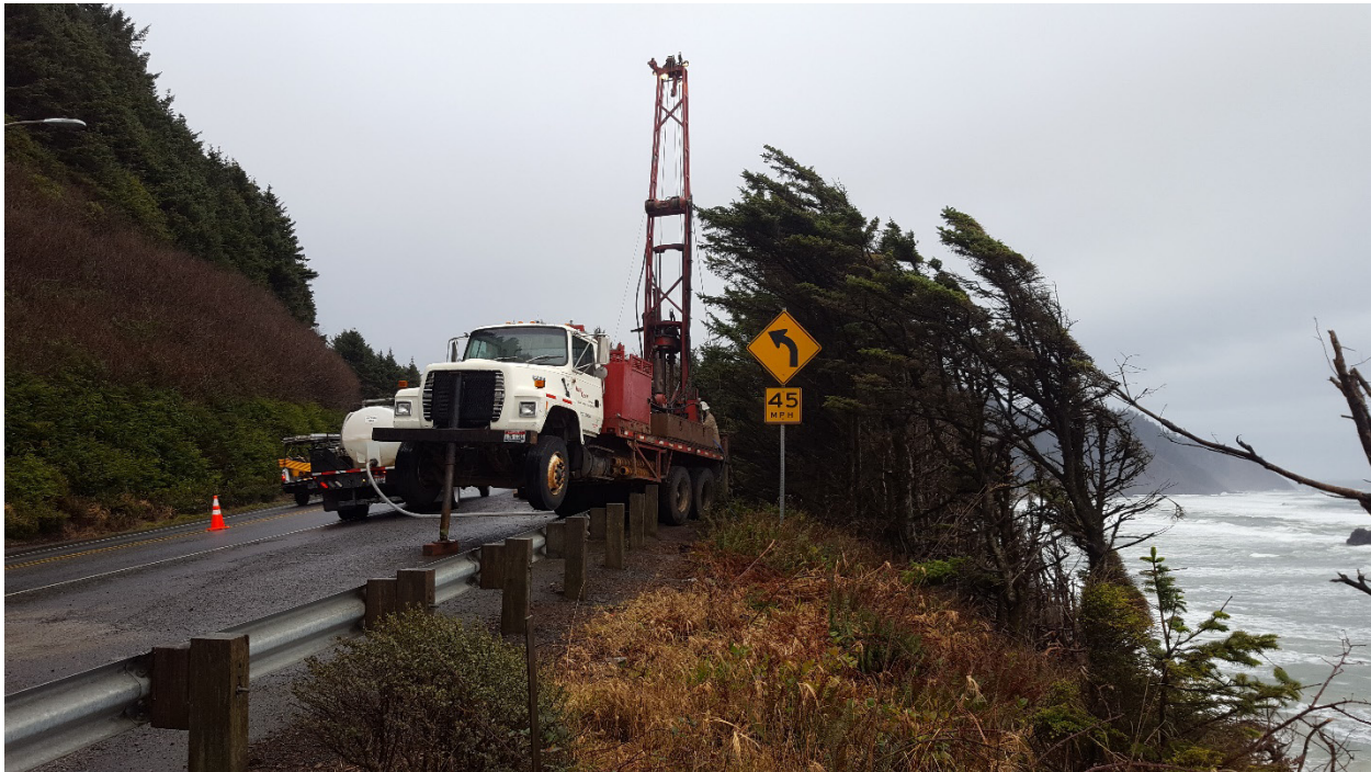
Figure 8.1: Drill rig actively drilling borehole for SAA MEM's installation at Arch Cape on January 20, 2017. Photograph Credit: Dr Michael Bunn.
