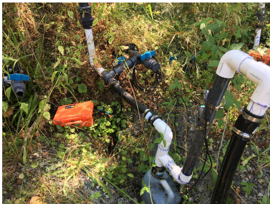
Figure 4.7 FloDar installed at Spangler field site, July 2022.
