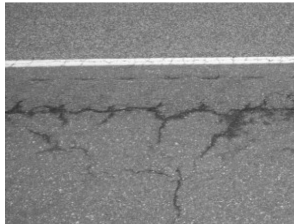
Figure 2.9: Fatigue cracking at milled rumble strips (Coffey and Park, 2016)
