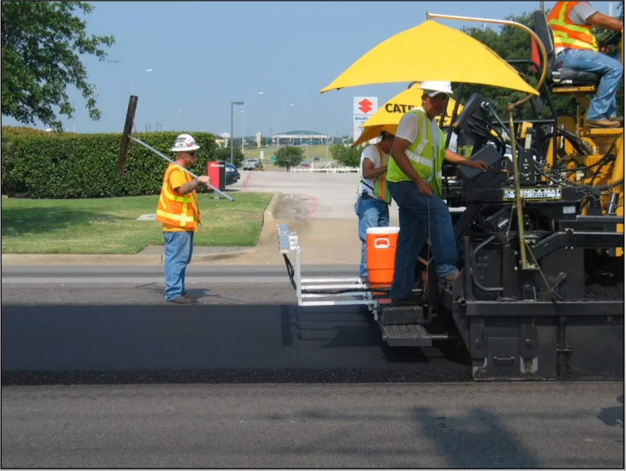
Figure 2.13: Straight vertical butt joint due to end gates down. ( https://www.youtube.com/watch?v=6NLURo8IBb4 )
