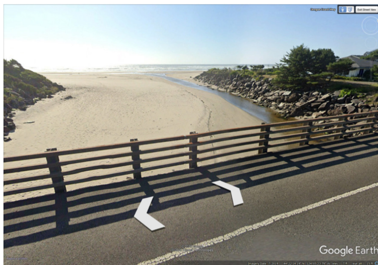
Figure 2.7: Riprap placed along the north and south stream banks and abutments at the bridge over Big Creek, MP: 160.15.
