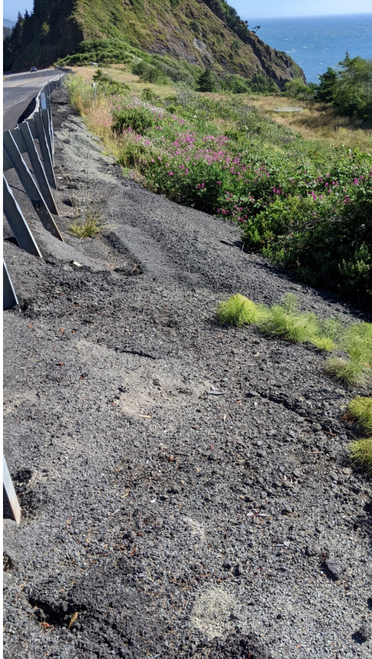
Figure 7.25: Shifts observed in guardrail and additional cracking (Photograph looking southeast, immediately west of the highway southbound lane & shoulder, July 2022)
