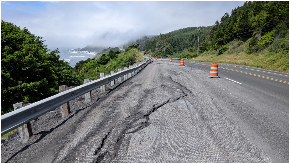
Figure 1.2: Localized slumping on Highway 101 looking north in the southbound lane at a site south of Port Orford, June 2022.
