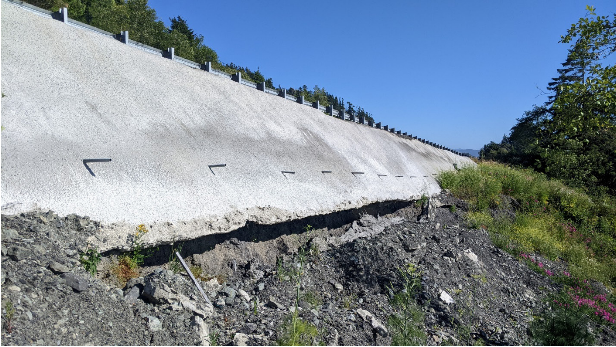
Figure 7.23: Undermining of a recently installed (2021) wall at the north end of Arizona Inn. (Photograph looking south east, July 2022)
