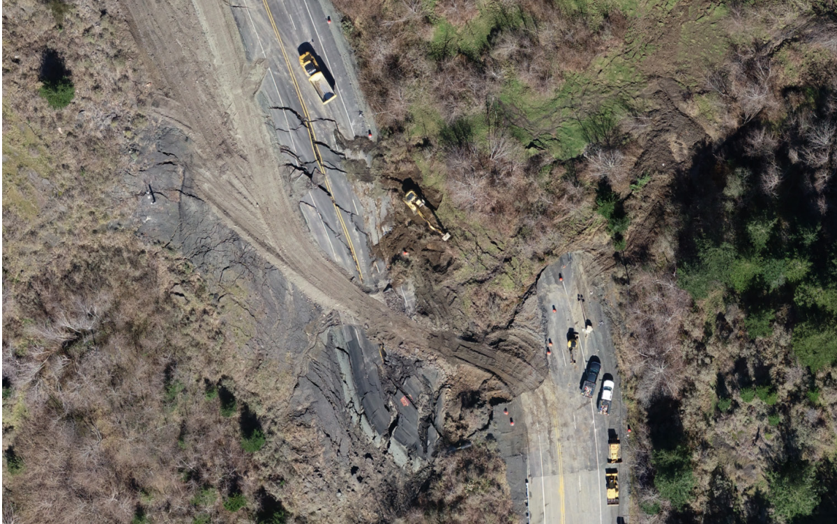
Figure 1.3: Damage to Highway 101 at the Hooskanaden landslide as a result of a major surge event in February 2019 (UAS orthophotograph obtained by Andrew Senogles and Richie Slocum).
