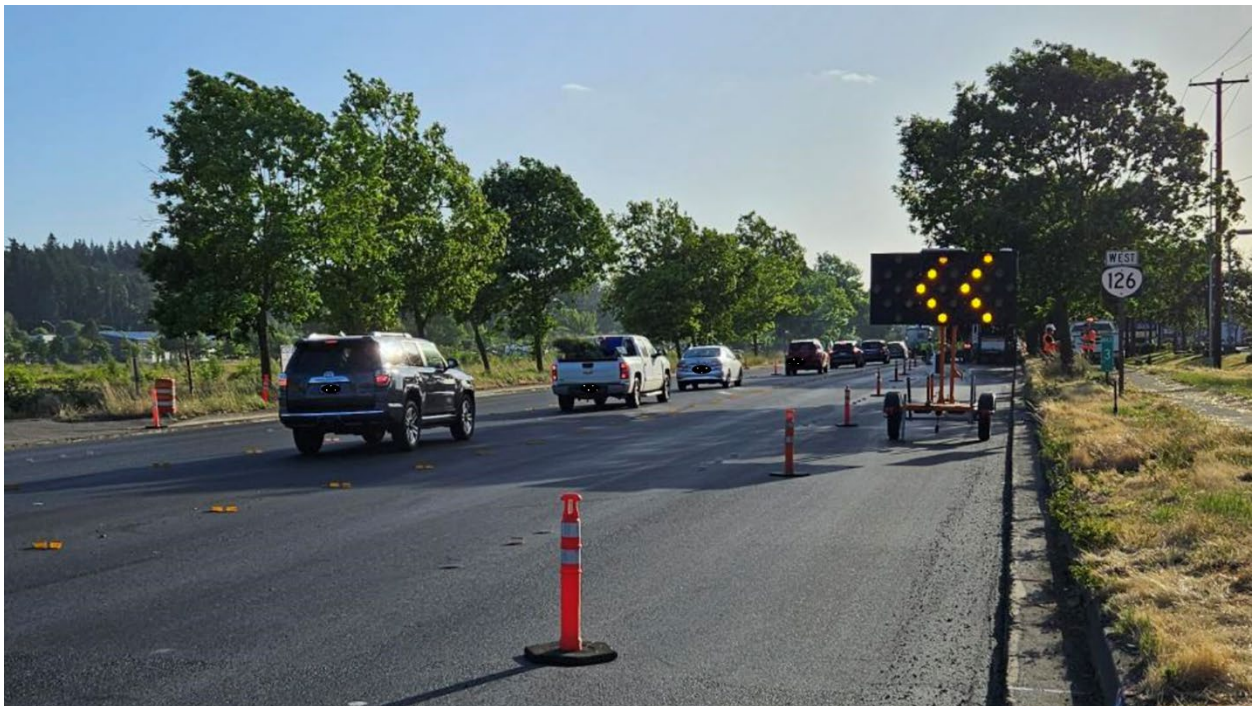
Figure 6.3: Smart Arrow Board Deployment
