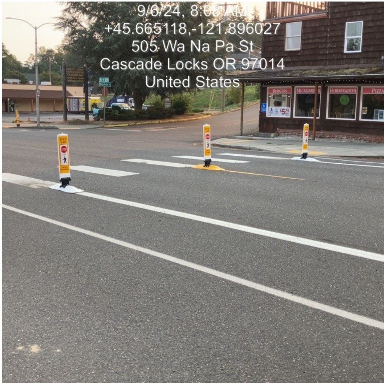
Figure 7.14 Wa Na Pa St. and Regulator St., Cascade Locks Stage 5 (R1-6a GTWY)
