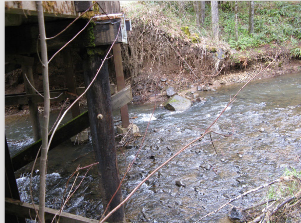
Kutch Road approach and interior footings failure
