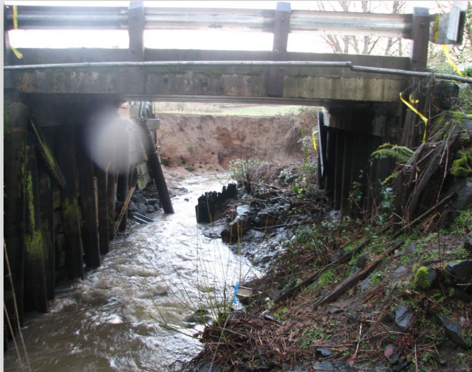
Ayers Creek Bridge failure
