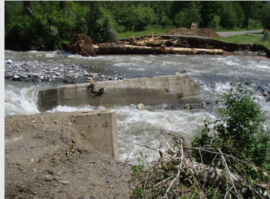
Holbrook Creek Road bridge failure
