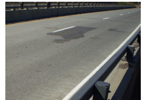
Large patches from previous repair
