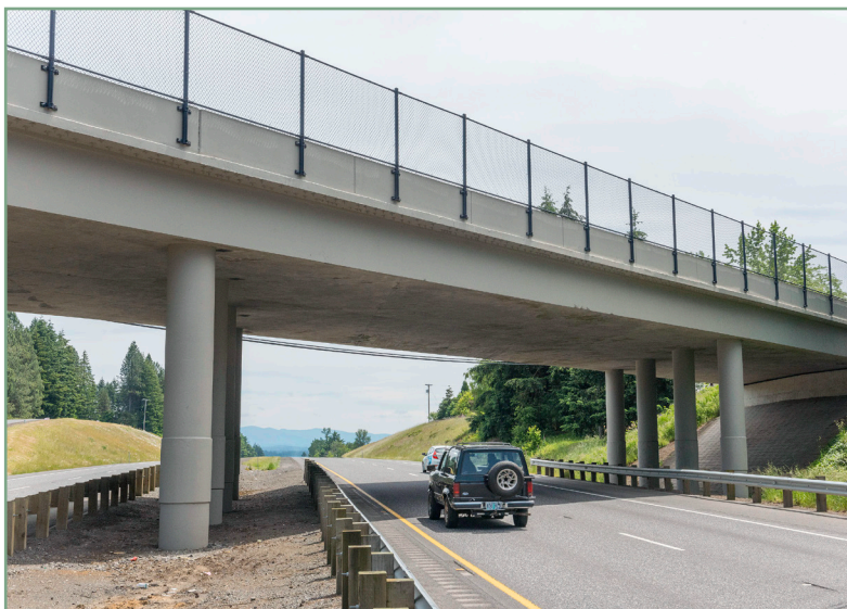
An example of protective screening similar to what ODOT will install on the Lake Road bridge over OR 224 in Milwaukie in early 2021.
