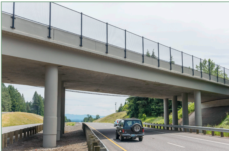
An example of protective screening similar to what ODOT will install on the NE 102nd Avenue bridge over I-84 and I-205 and the railroad access bridge just to the east.
