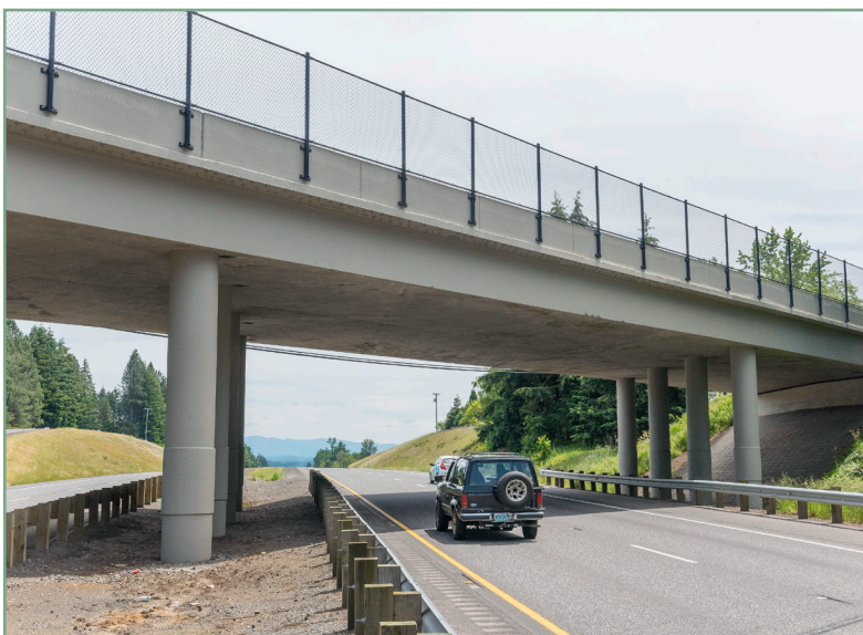
An example of protective screening similar to what ODOT will install on the north side of the OR 43/South Macadam Avenue ramp to U.S. 26/City Center in South Portland.
