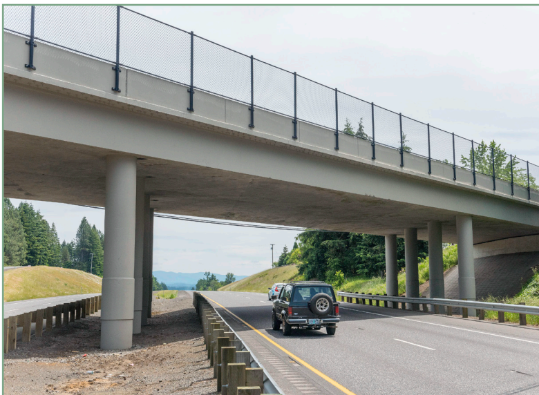
Protective screening will help improve safety on and below the Lombard St. bridge over I-5. We will also install new railing on both sides of the bridge.
