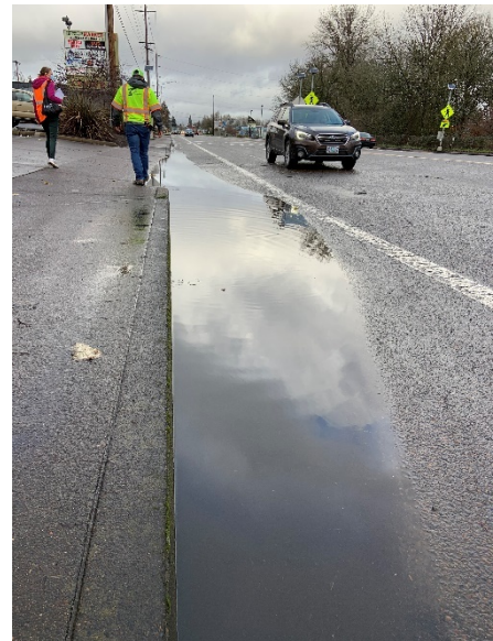
Standing water spans the bike lane near Mill Race Bridge
