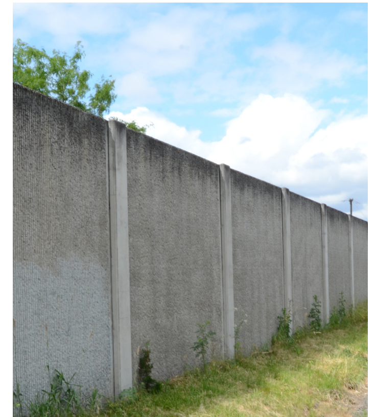
This is an example of what a post and panel sound wall looks like.
