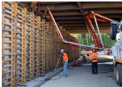
Crews work under I-5 to build a new structure over SW 26th Avenue in Portland.
