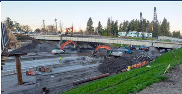
Crews demolish the SW Hall Boulevard overpass in Tigard during a weekend highway closure.
